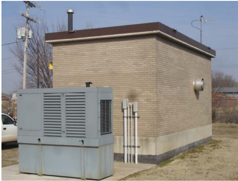
This photo shows the Brush Creek pump station , located on 40 th Street. This pump station has (2) 47 HP, 520 gpm pumps. The pump station is set up for (3) pumps. This pump station has a standby generator located on site and is on a SCADA alarm system.
