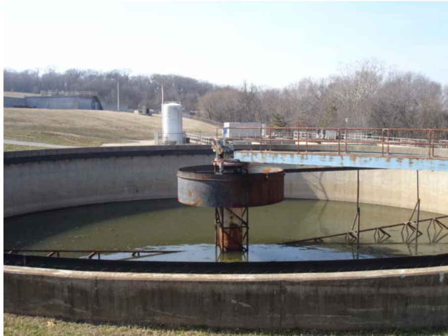
This photo shows one of the two old final clarifiers that is used as an EQ basin for excessive storm water.
