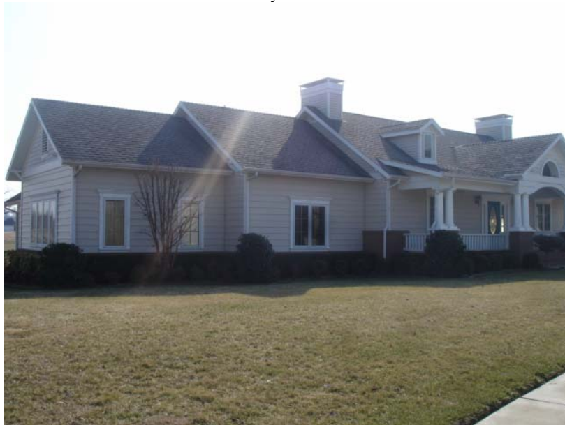
This photo is of the Har-Ber pump station , located on Ireland Street in the Har-Ber Meadows subdivision. The pump station is located within the "shell" of this home. This pump station has (2) 47 HP, 350 gpm pumps. The pump station is set up for (3) pumps, the 3 rd being 88 HP, 700gpm. This pump station has a standby generator located on site and is on a SCADA alarm system.
