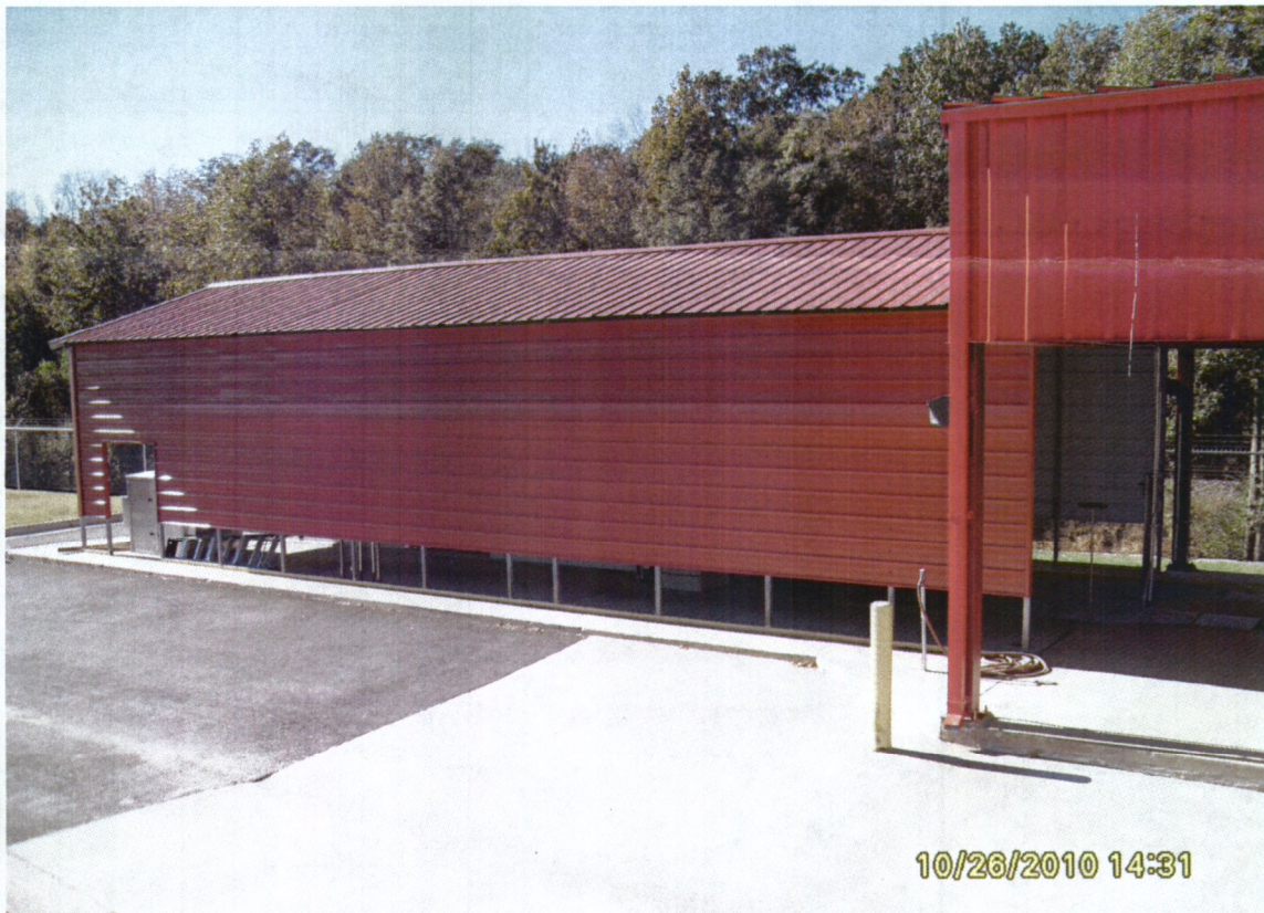
Enclosure Siding to Control Algae Growth @ Plant Effluent Meter and Sample Collection Station
