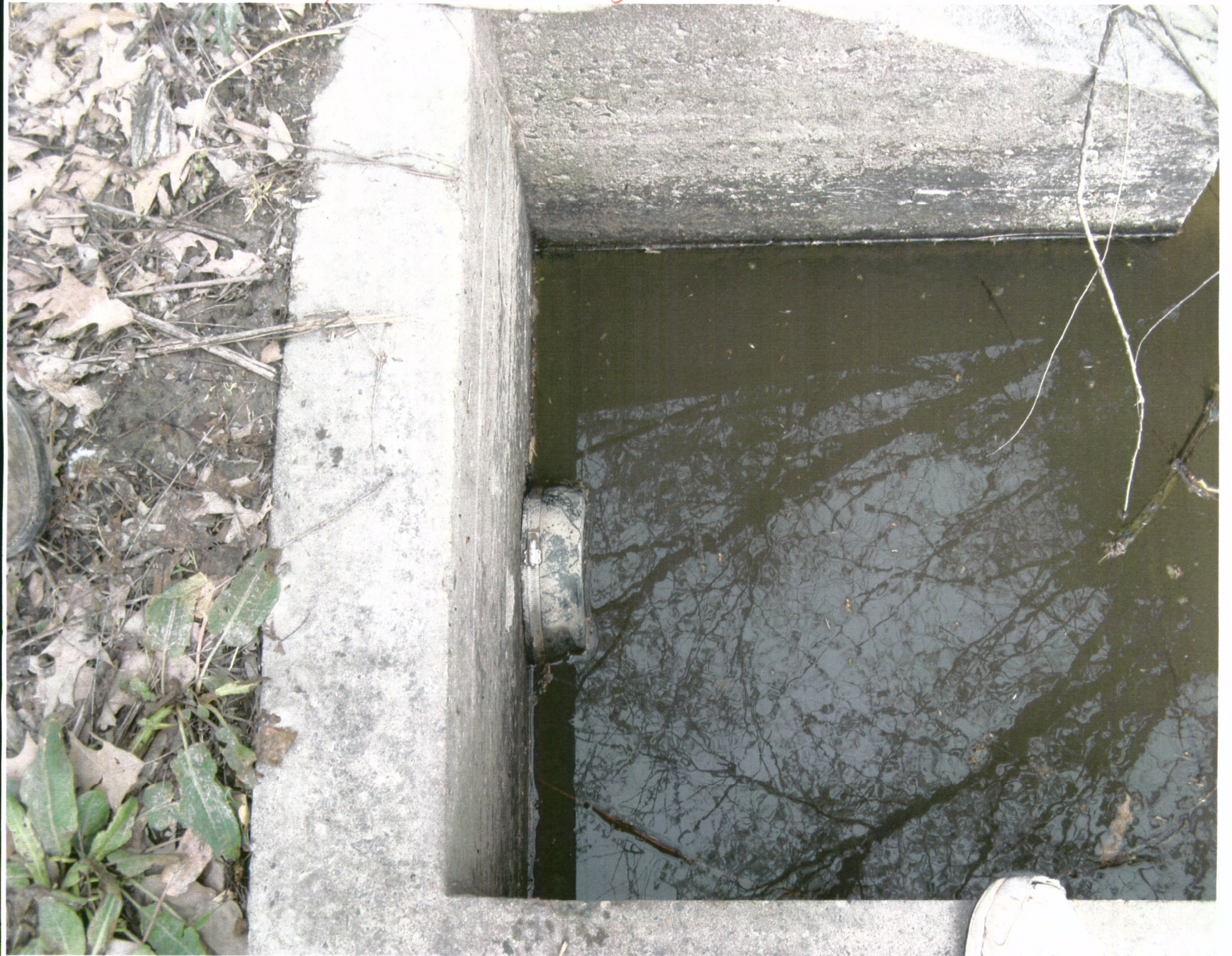
Photo # 2 - Discharge Pipe Cap
