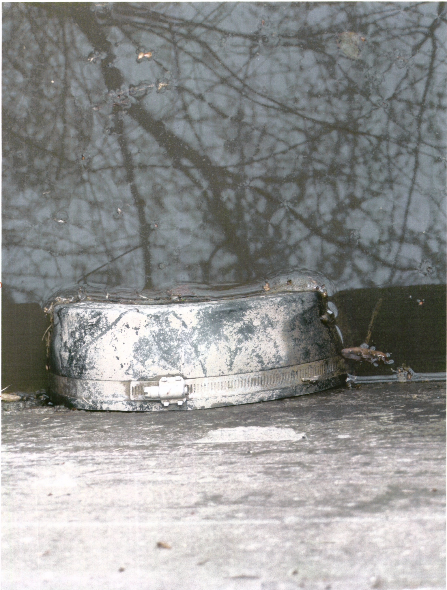
Photo #3 Discharge Cap Reinforcement
