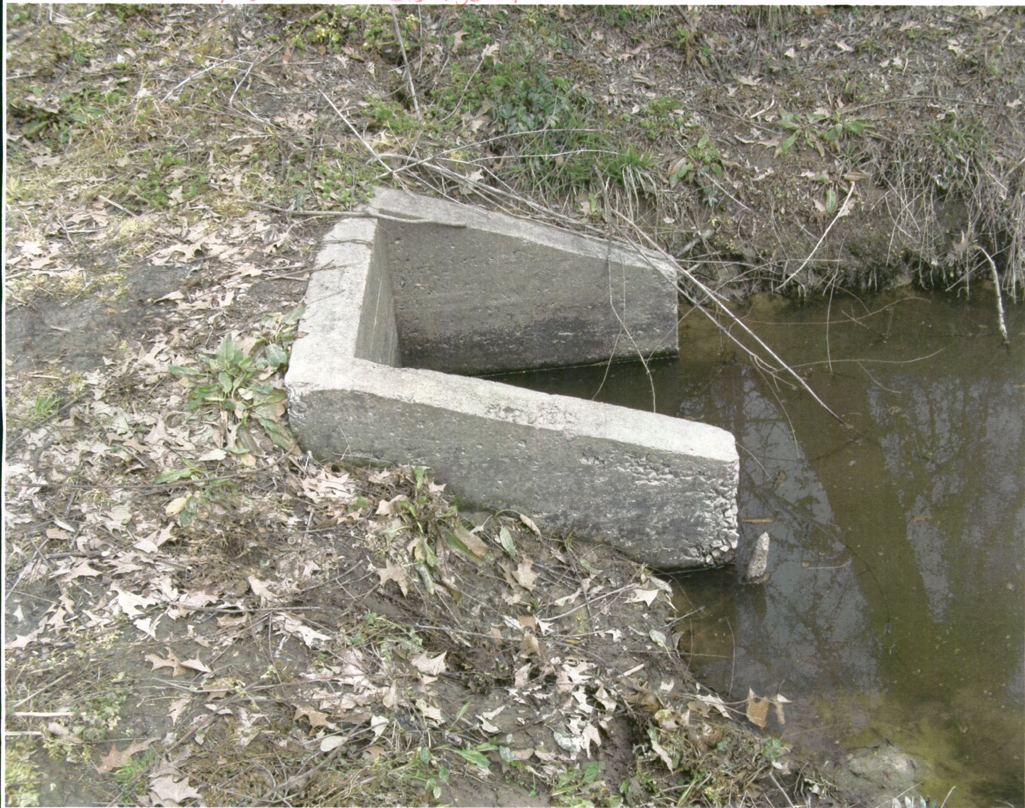
Photo # 1 - Discharge Pipe
