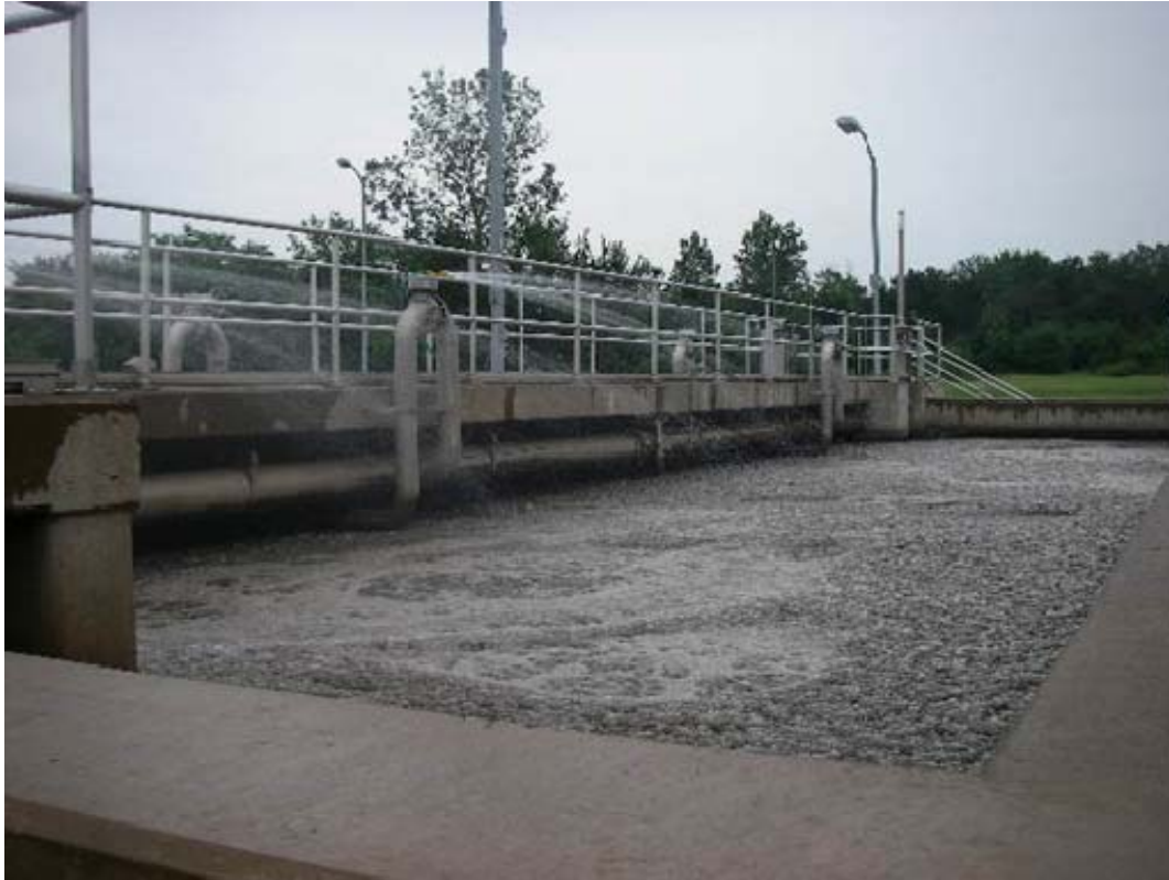
Activated sludge basin
