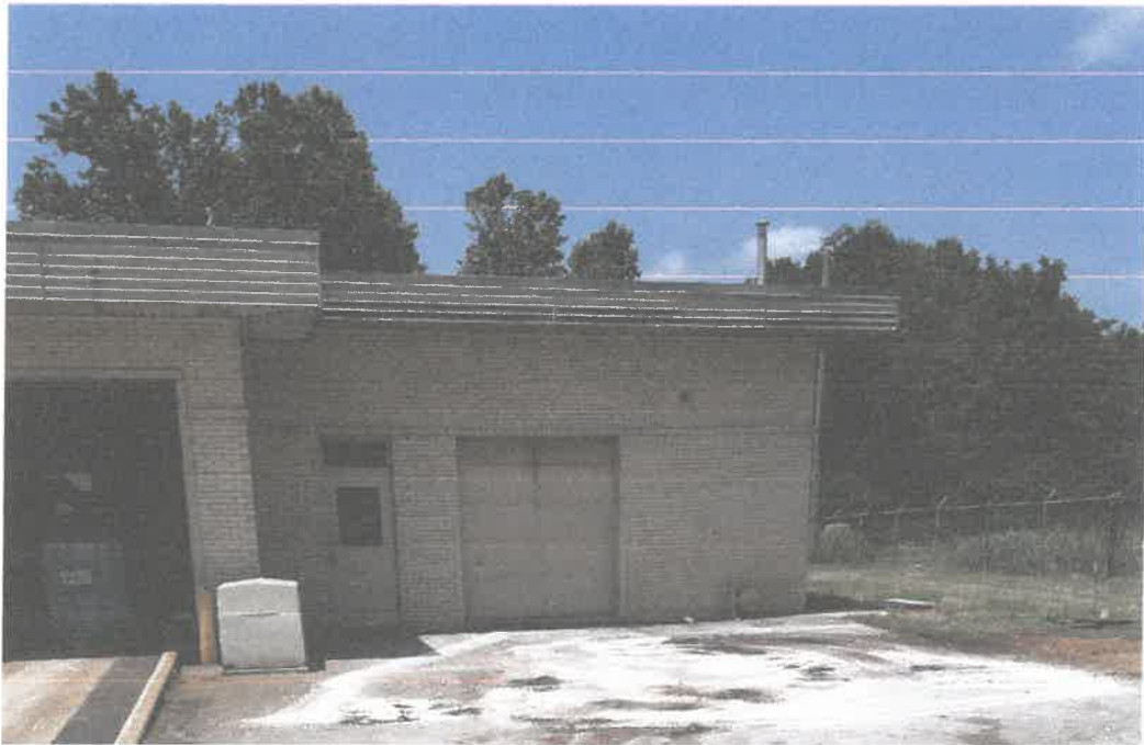
Picture 8 Tote Storage Area Cleaned Removed Old Tanks and Applied Oil Dry Compound.
