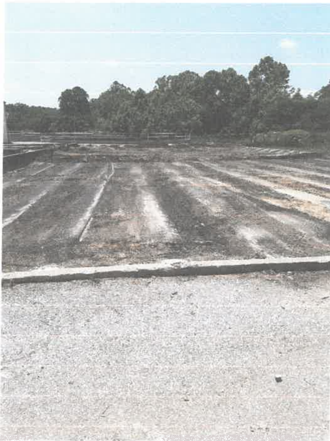
Picture 5 Sludge Drying Beds Cleaned Vegetation Removed
