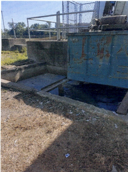
1) South Pump Station
