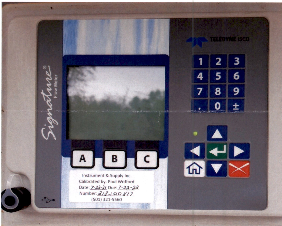
Effluent Meter Calibration July 22, 2021 Instrument & Supply Paul Wofford
