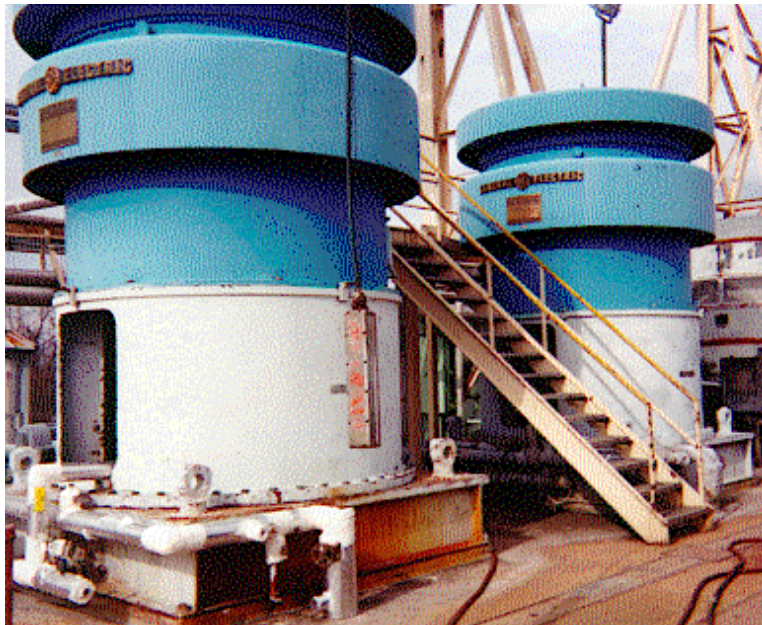
Figure 2.3 Circulating Water Pump Motor
