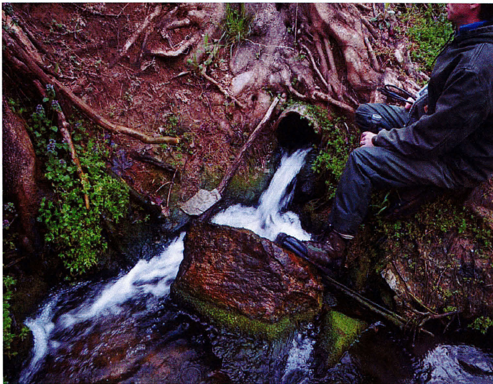
Photo A.10. YWWTP Outfall 001 on April 3, 2013.
