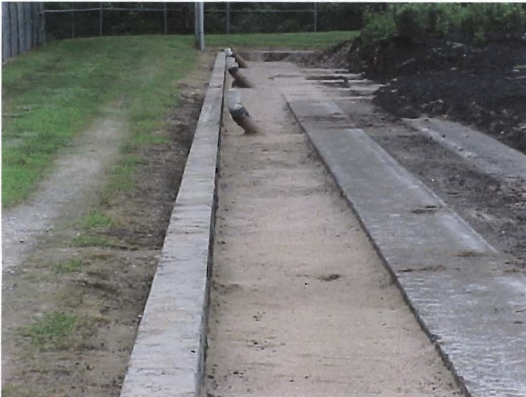
Figure # 1: Looking south on the east side of the sludge storage bed
