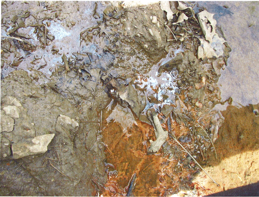
Close Up of North End of Encasement Looking Down Where Groundwater is Appearing Photo Taken 21 April, 2009
