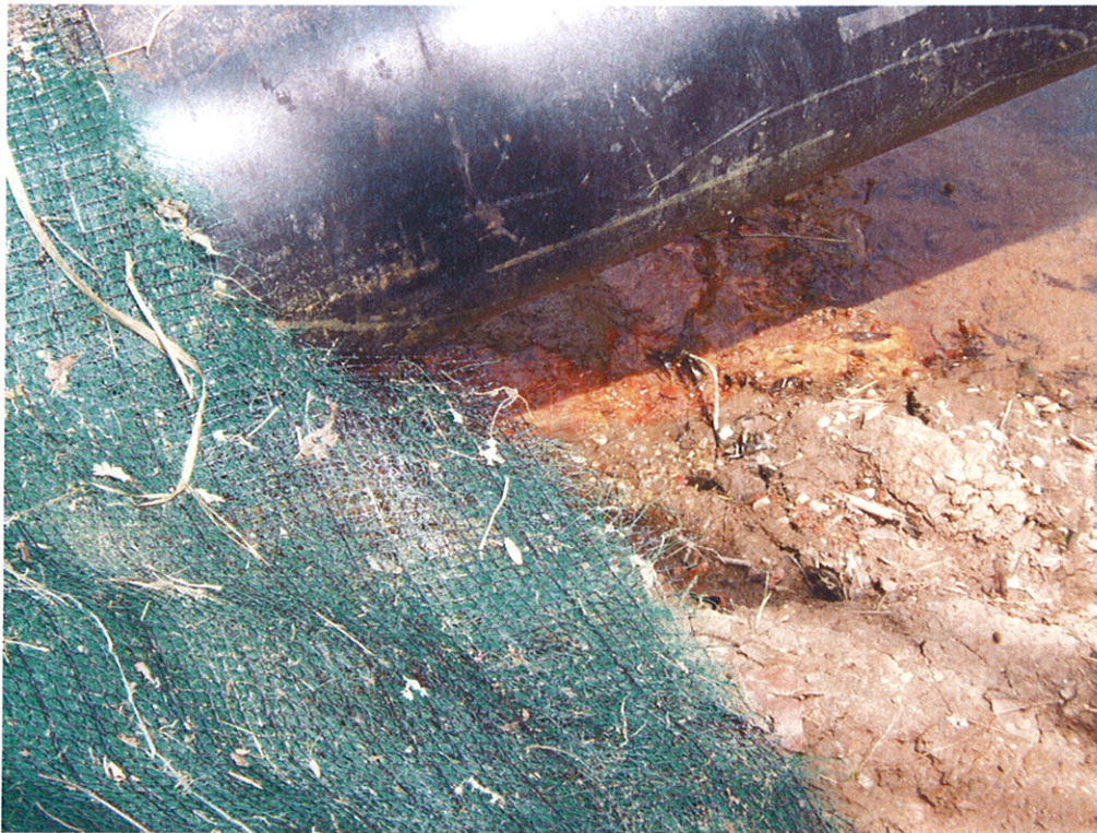
North End of Encasement Where Groundwater is Appearing Photo Taken 21 April, 2009
