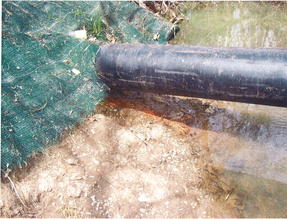
North End of Encasement Where Groundwater is Appearing Photo Taken 21 April, 2009
