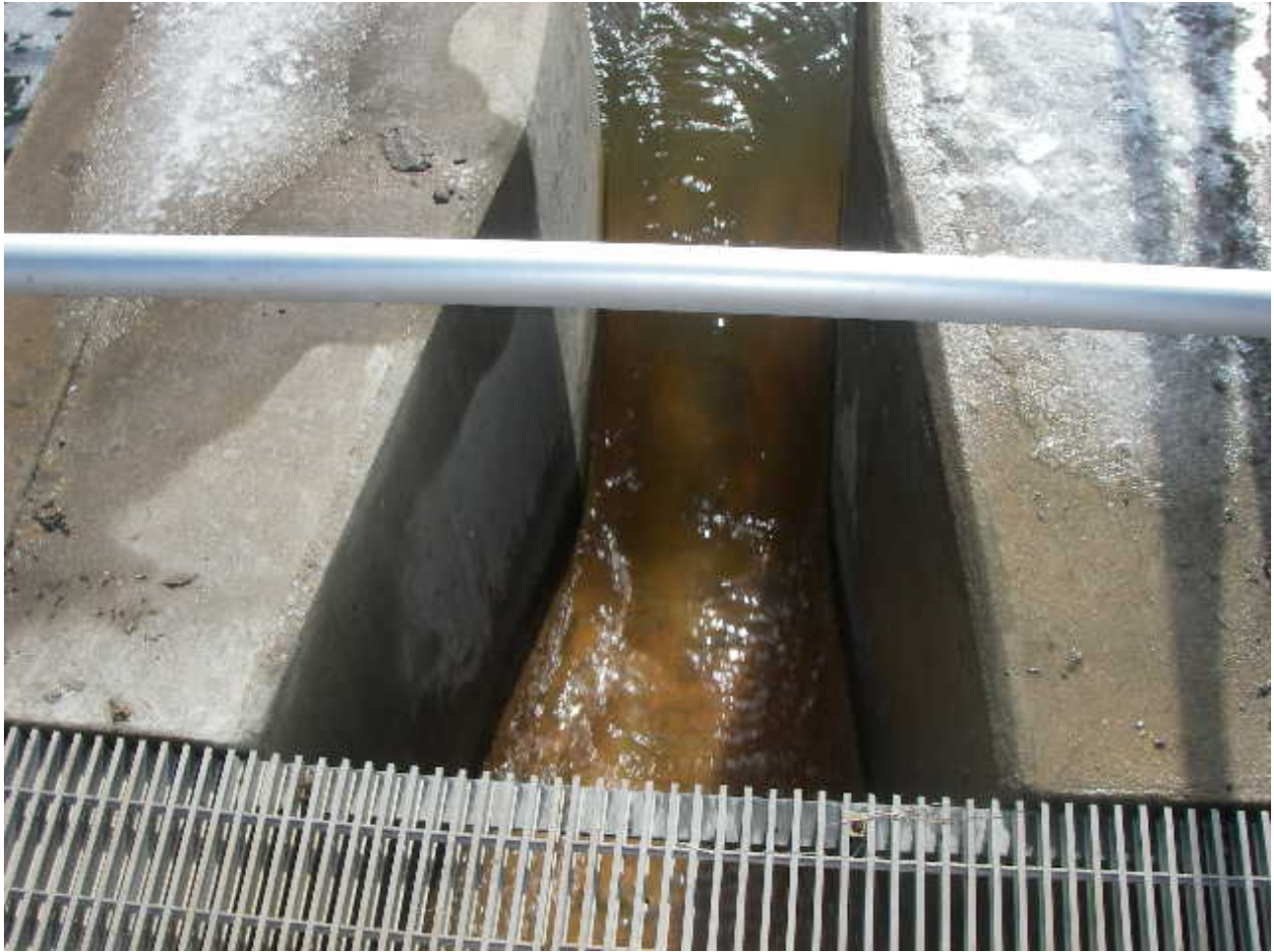
Photo of Parshall flume at the Harrison POTW showing clear effluent on 1/30/09
