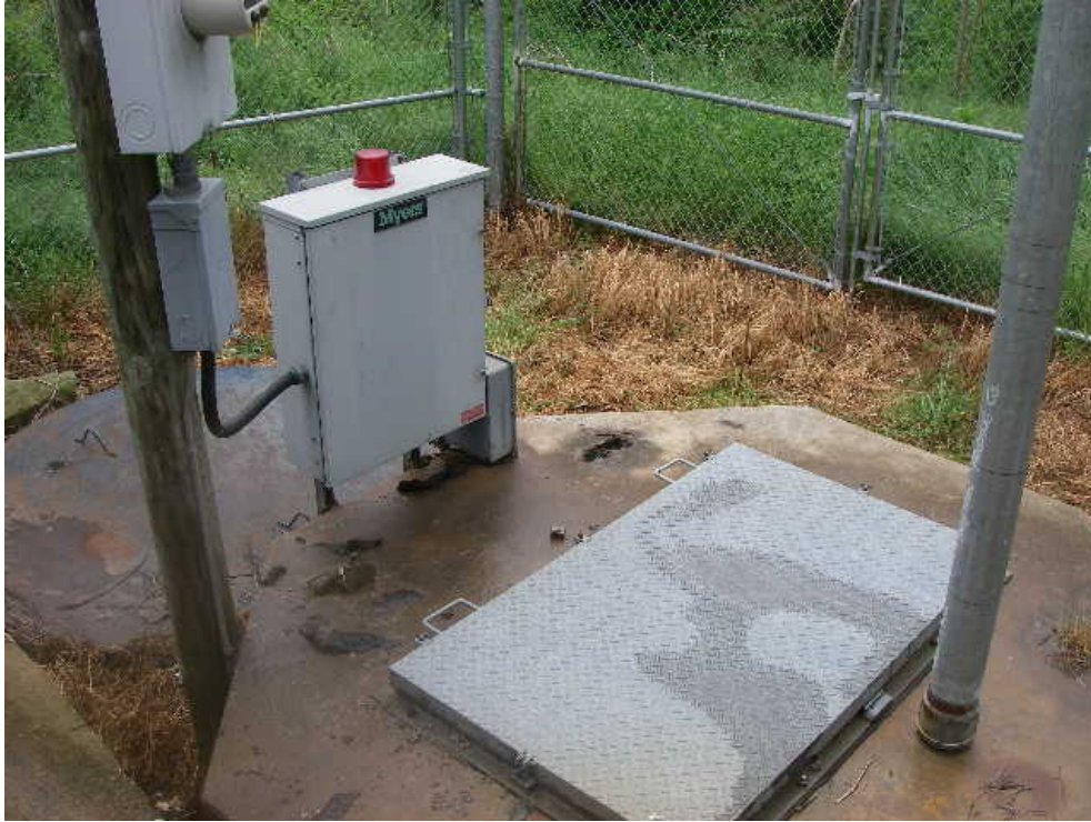
Lift station which failed
