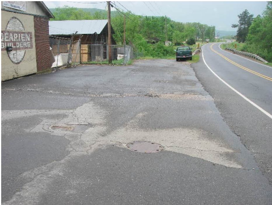
Manhole which overflowed as result of lift station failure
