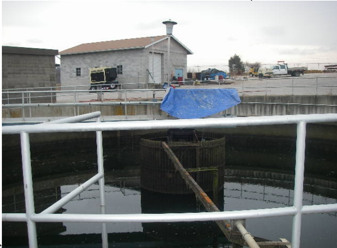
Photo of North Clarifier which was not in service at time of inspection due to motor failure
