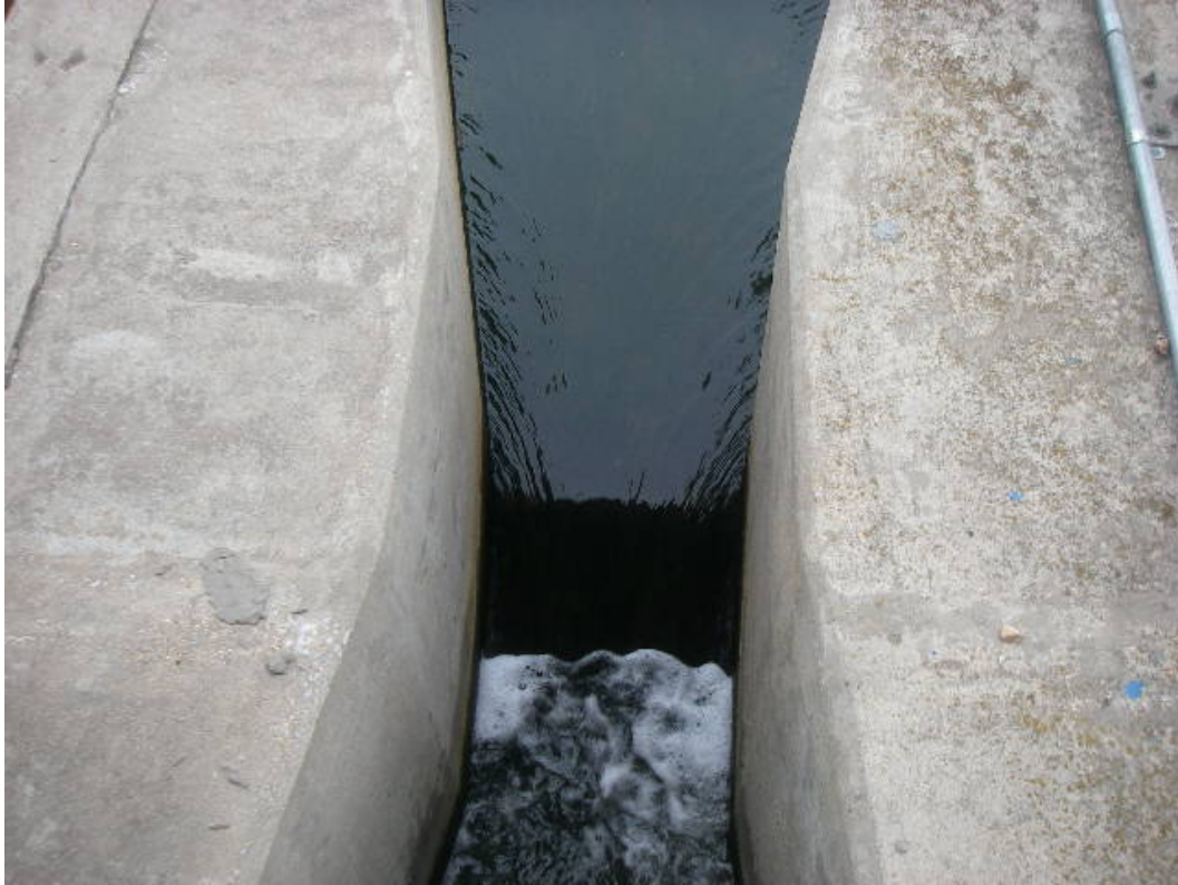
Photo of Parshall flume showing effluent that appeared to be of good quality on 1-19-2011
