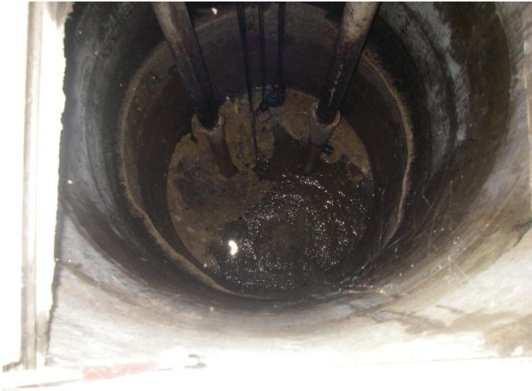
Ray Road Lift Station wet well
