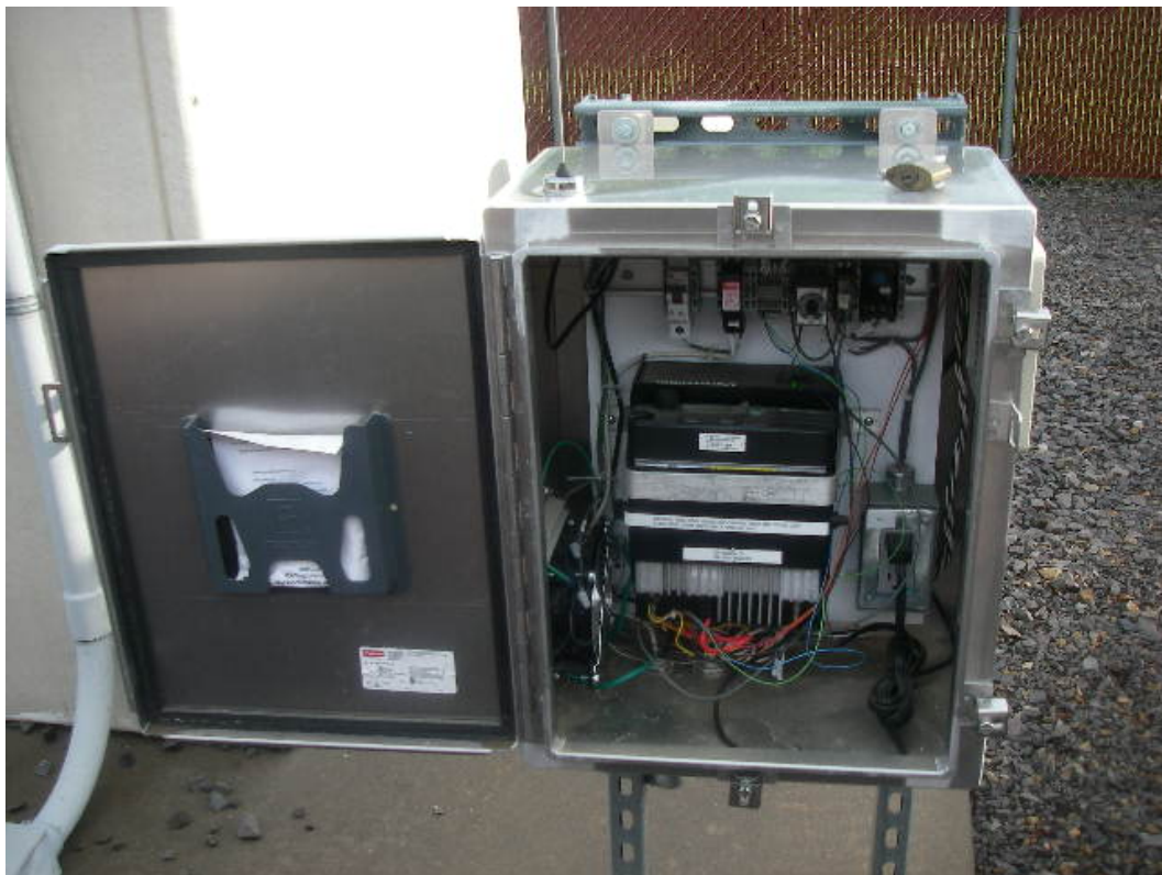
Ray Road Lift Station SCADA call box
