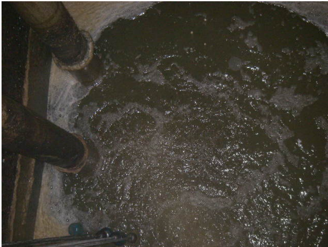
South Park Lift Station wet well
