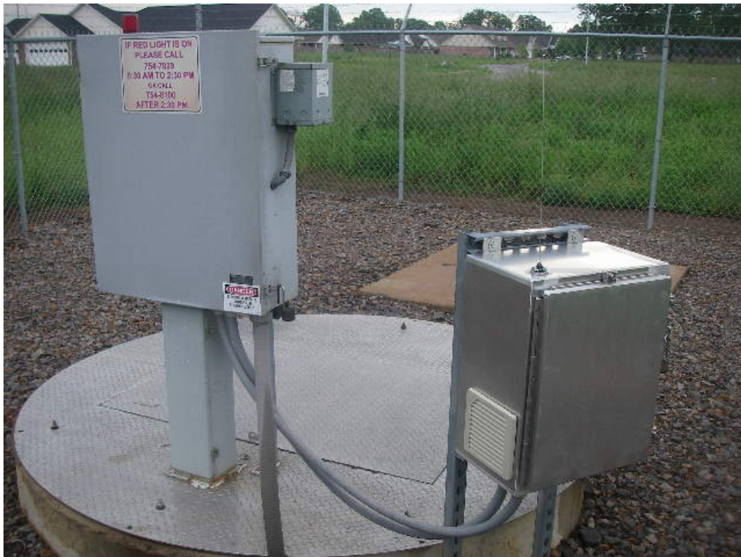
Stegall Lift Station SCADA call box and electrical control panel
