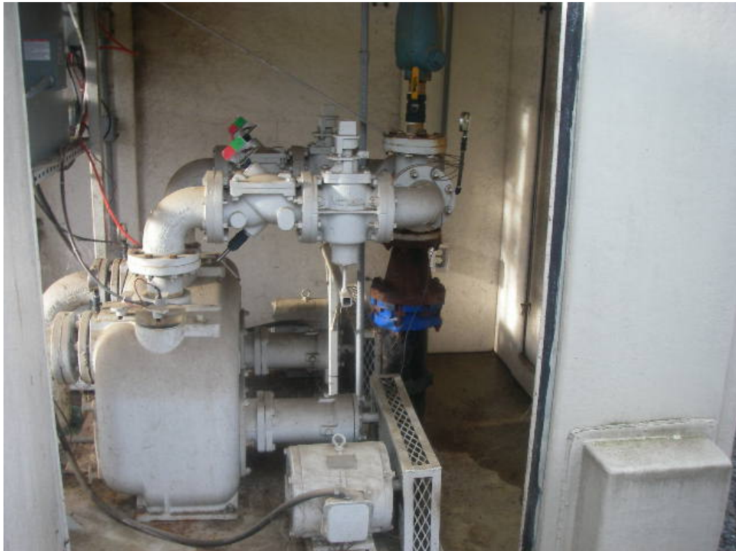
Ray Road Lift Station
