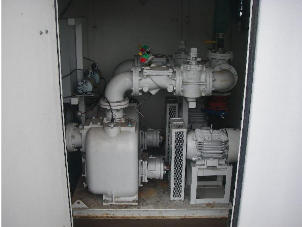
South Park Lift Station
