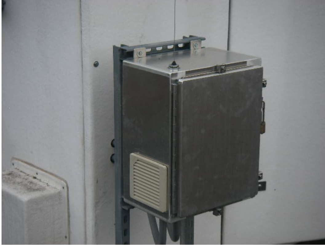
South Park Lift Station SCADA call box
