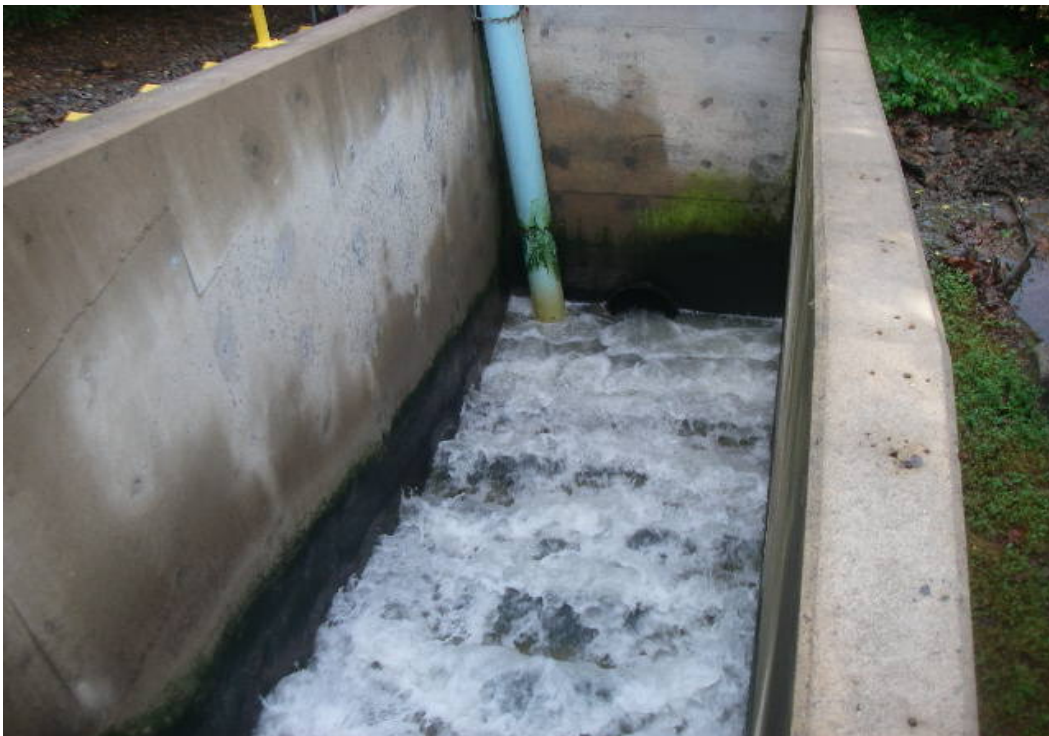
Post aeration for Outfall 001
