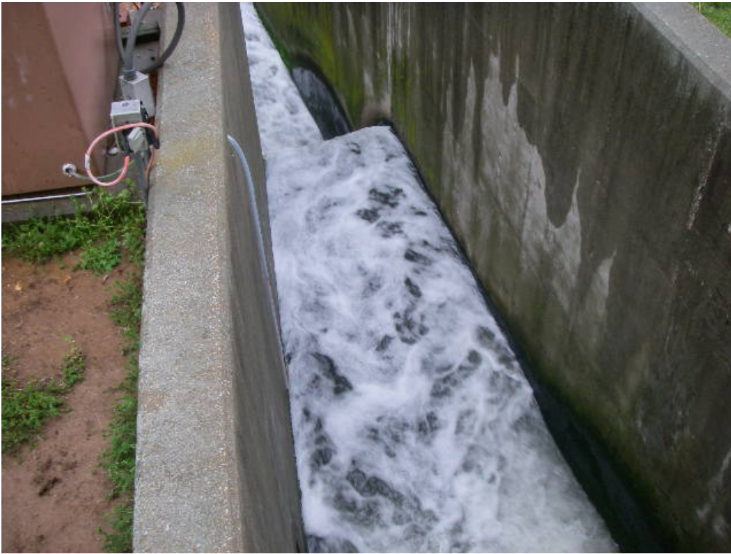
Post-aeration cascade for Outfall 001
