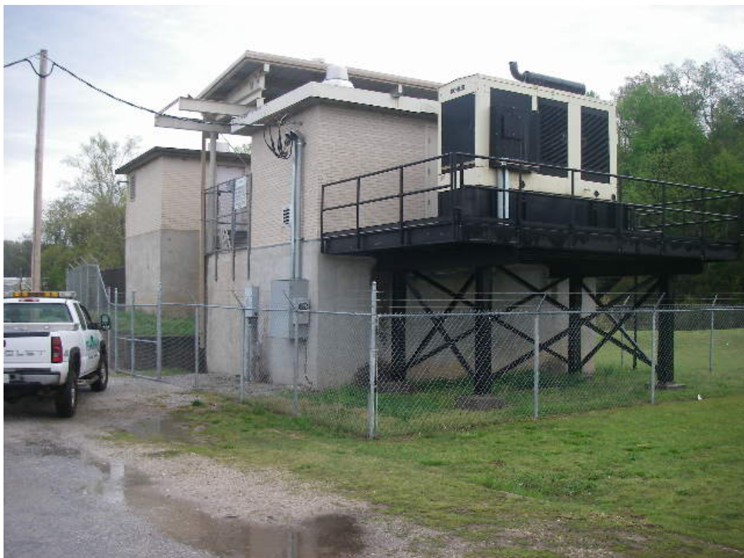
Main lift station with generator
