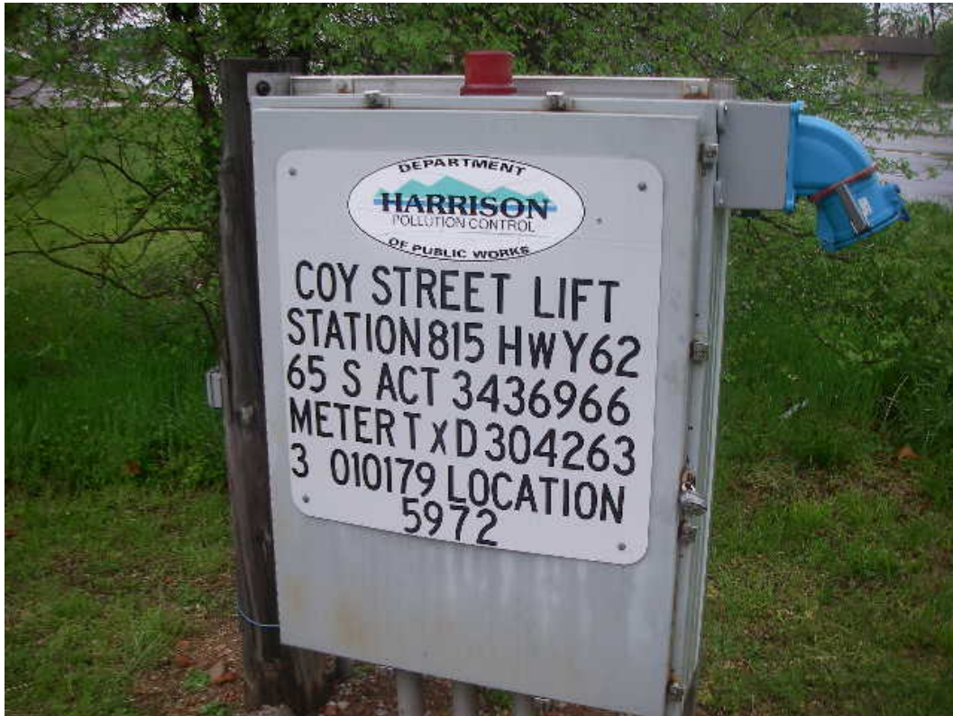
Coy Street Lift Station control panel
