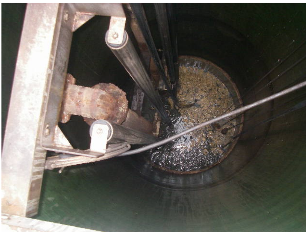
Wellington Lift Station wet well
