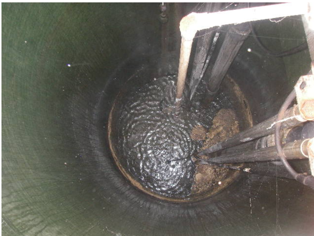
Brewer Street Lift Station wet well
