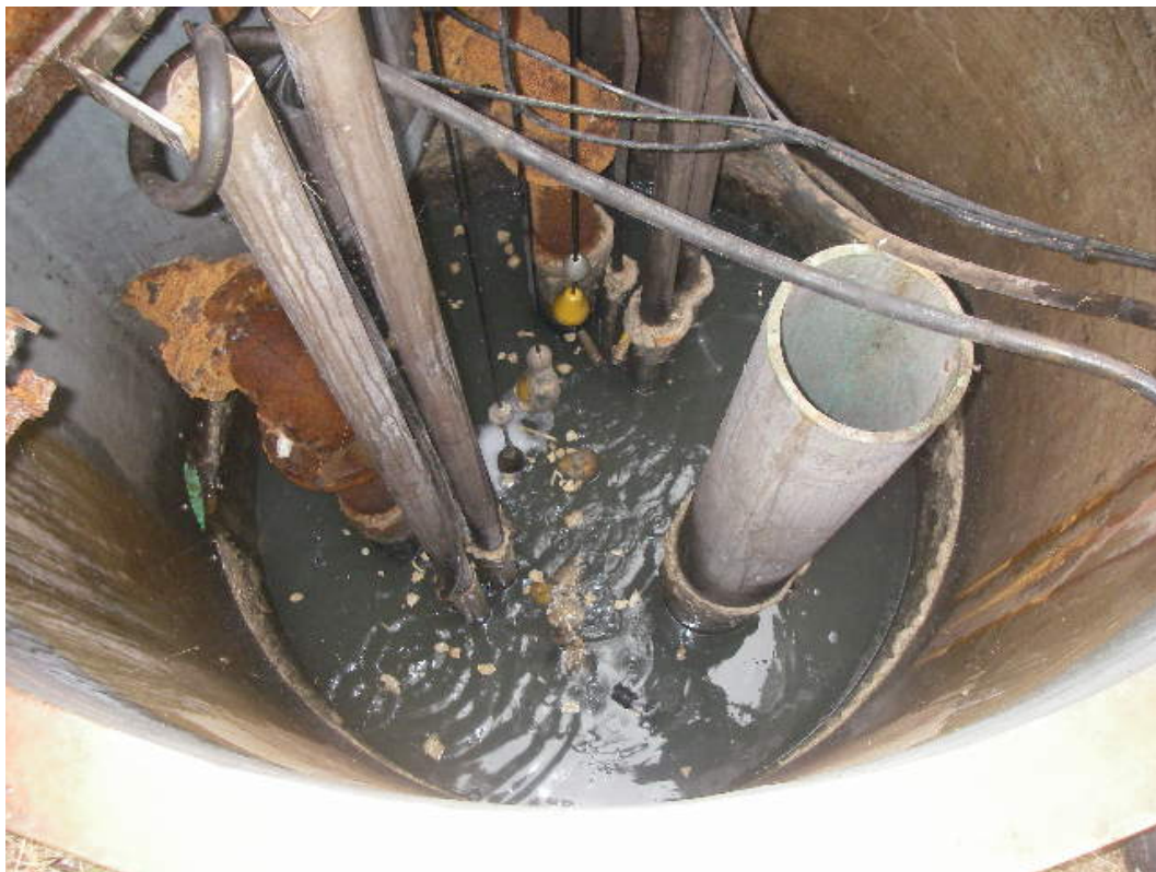
Coy Street Lift Station wet well
