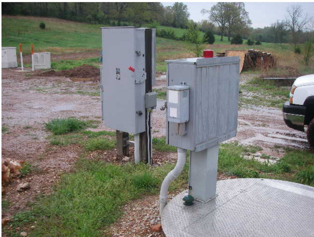
Wellington Lift Station
