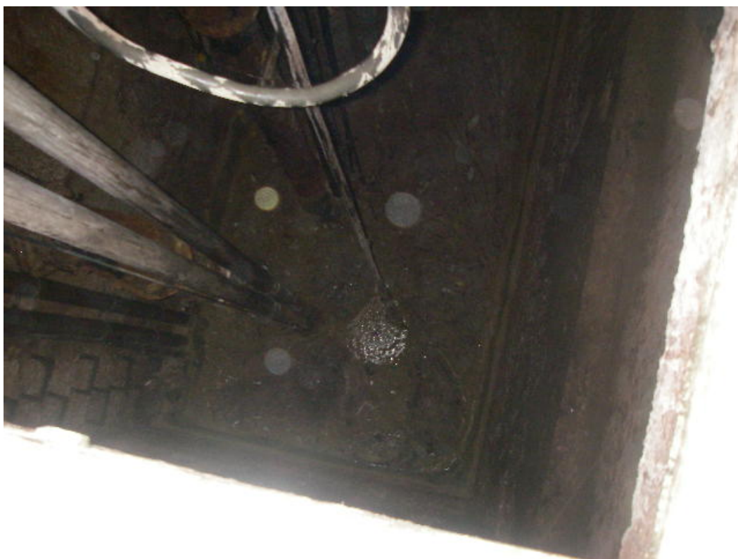
Main Lift Station wet well
