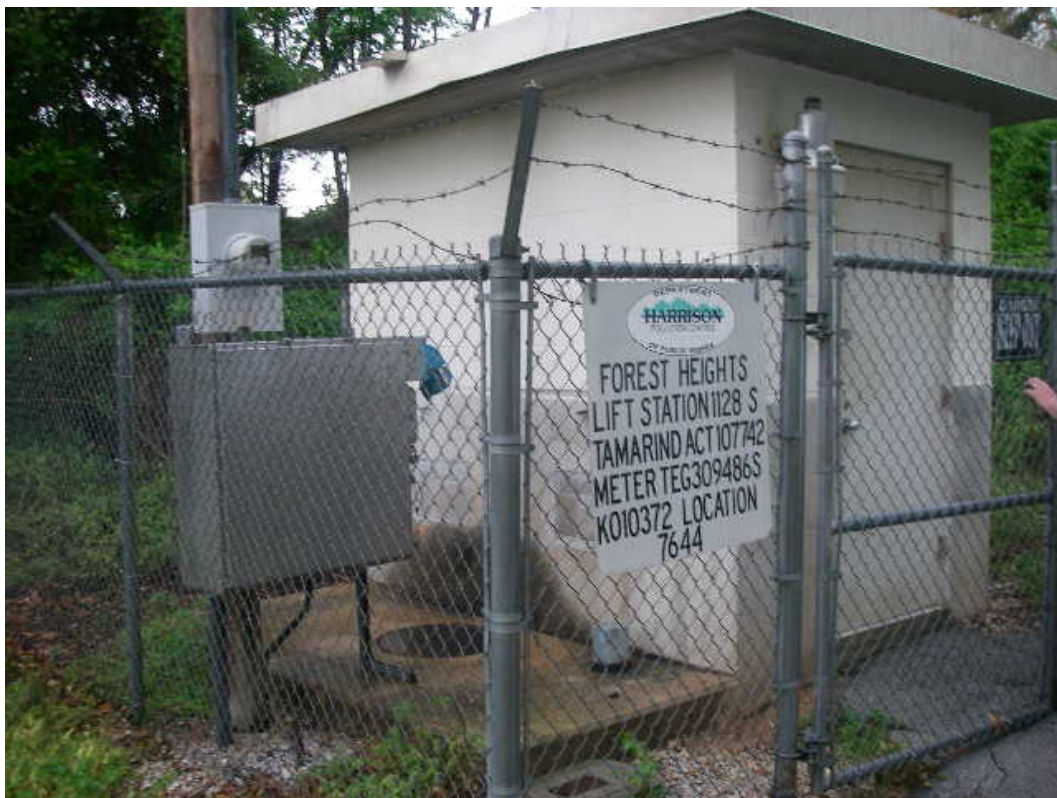
Forest Heights Lift Station
