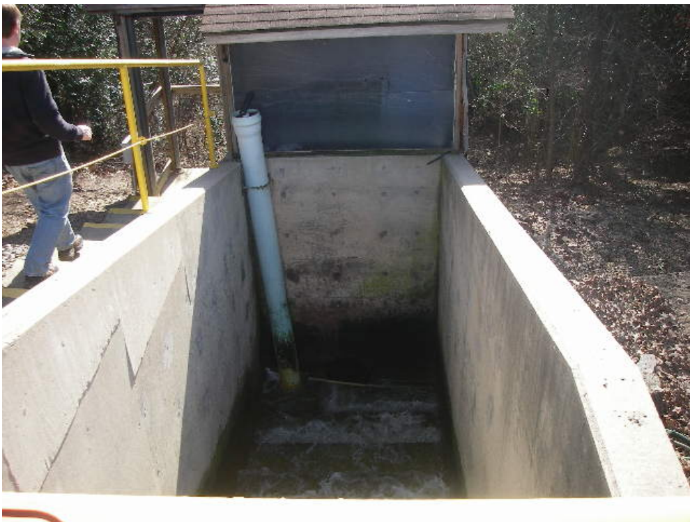
Post-aeration for Outfall 001
