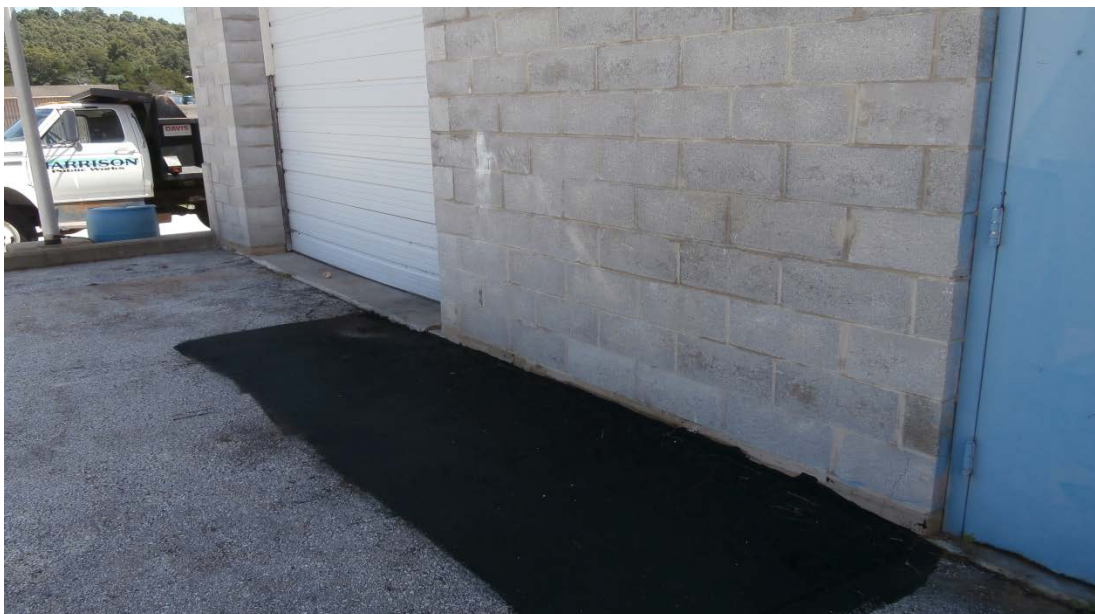
Photo #2 Unsealed barrels and spill/leak constituents exposed to stormwater – AFTER Asphalt sealant used to seal oil stains.
