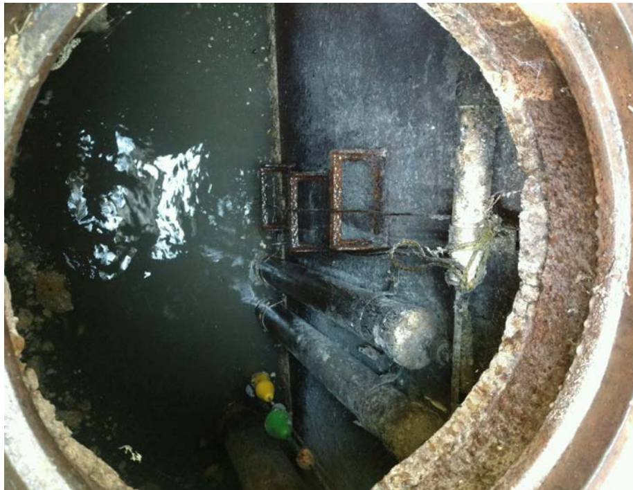
Photo # 12 Wet well of Forest Heights Lift Station; solids/grease moderate. AFTER
