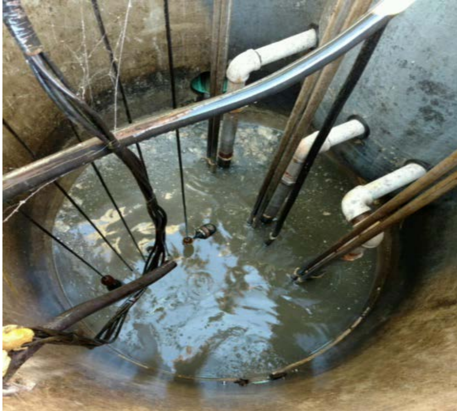
Photo #4 Wet well of Meyers Lift Station; solids/grease high. AFTER
