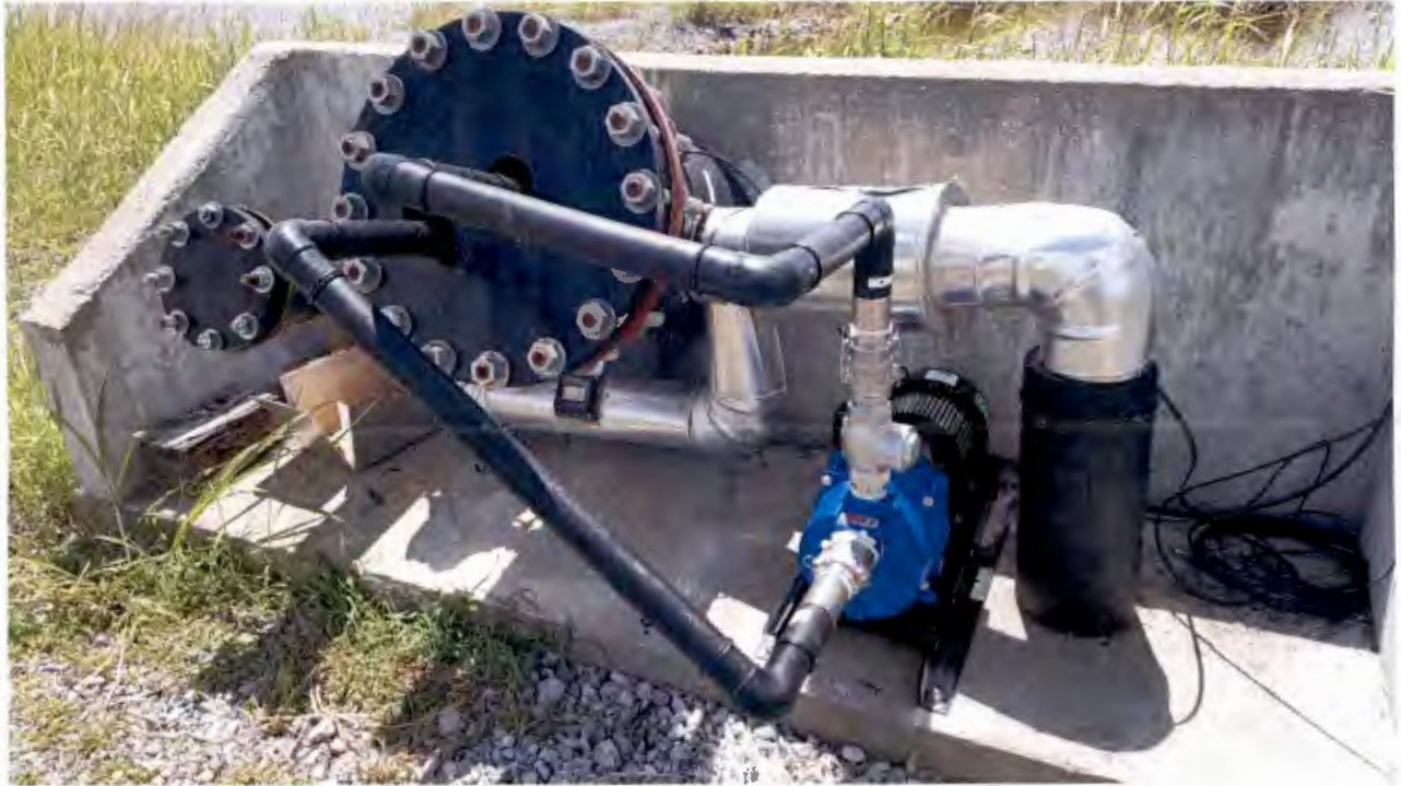
Entergy Arkansas, Inc. - Independence Plant Permit No.: 0200-S3N-R2 AFIN: 32-00042 Cell 15 – Installed leachate collection sump pump View to the west 6/22/2017
