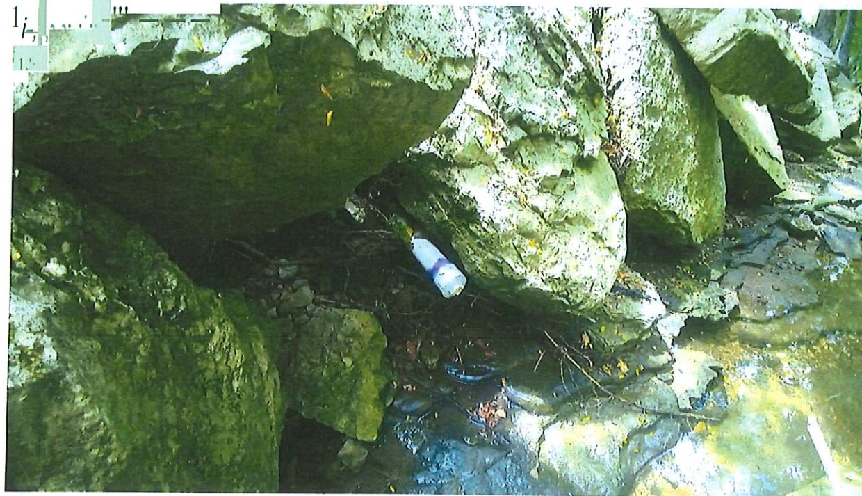
This is a picture of the pipe that was referenced by Ms. Nautiyal as photo #3 which was discharging water.
