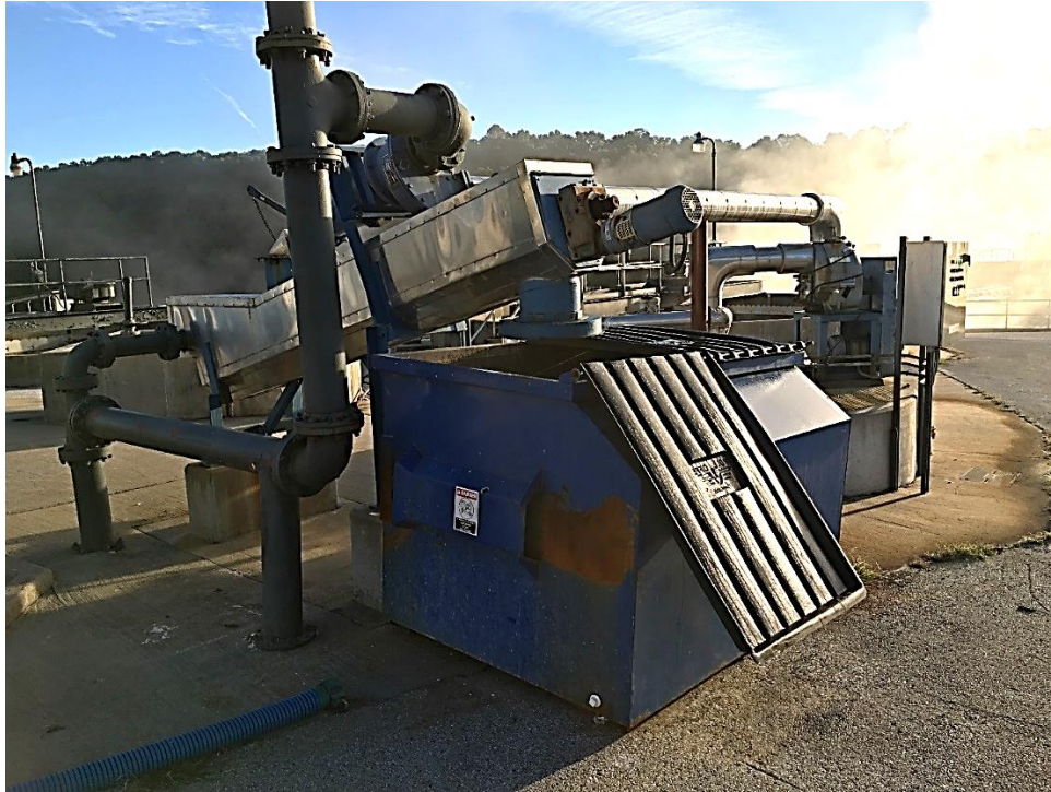
Photo 1 – Grit screening collection container
