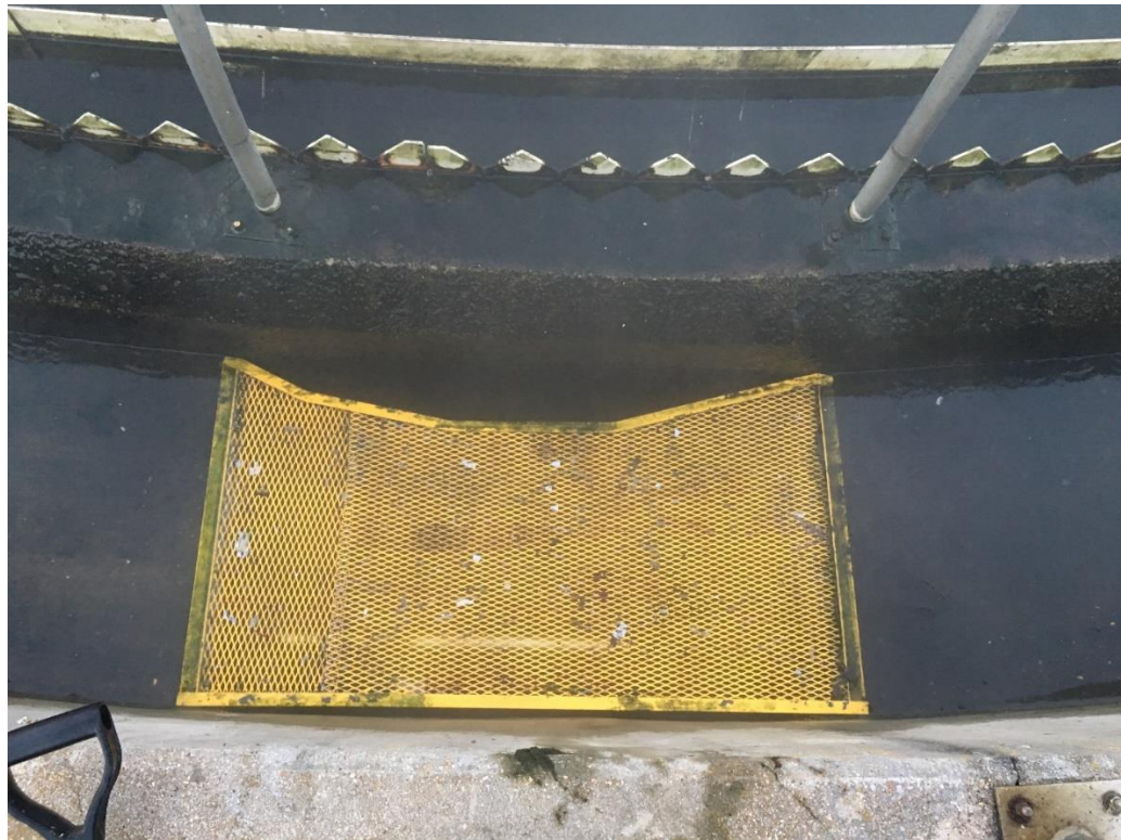
Photo 9 – Catch screen at final clarifier discharge.
