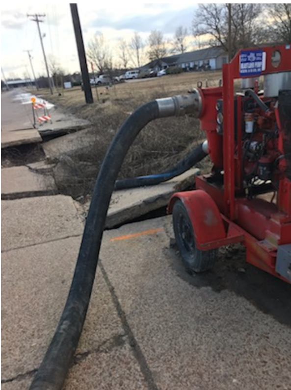
Collection System-Woods (Photo1)
