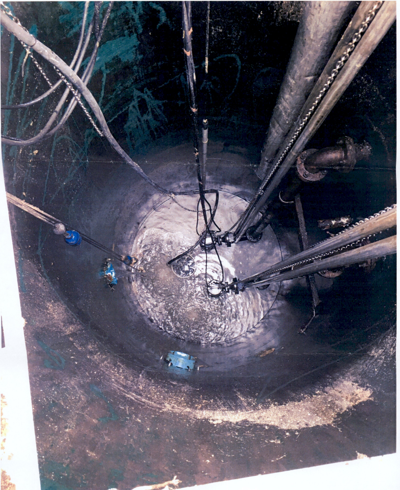
Grant Lift Station
