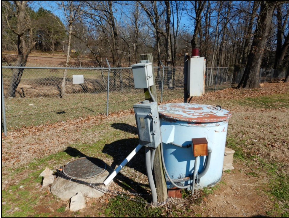
Photograph 1. Influent pump station dry well access hatch and wet well manhole cover.
