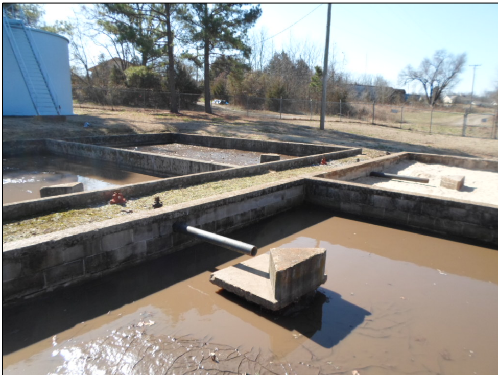
Photograph 10. Sludge drying beds and digester (background).
