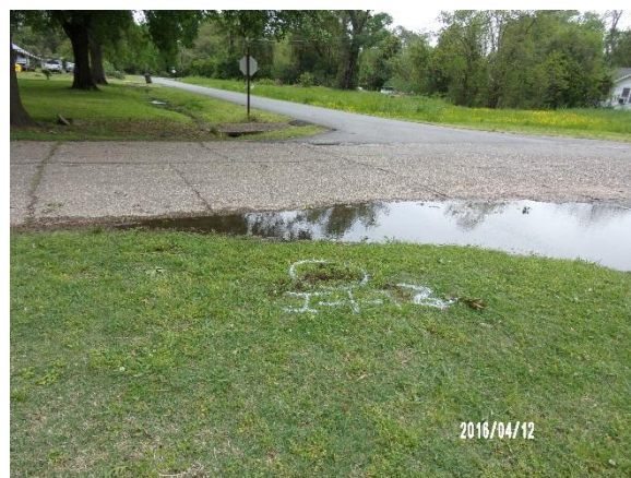
Figure 9 -Example of low manhole lid
