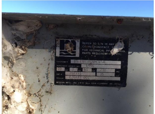
Figure 6 -Existing pump station info tag
