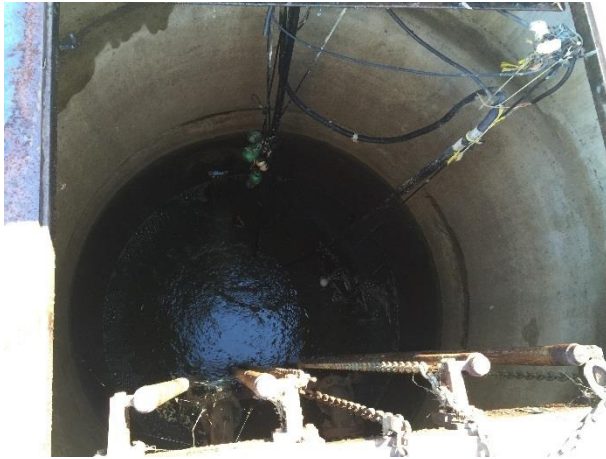
Figure 5 -Interior view of existing pump station
