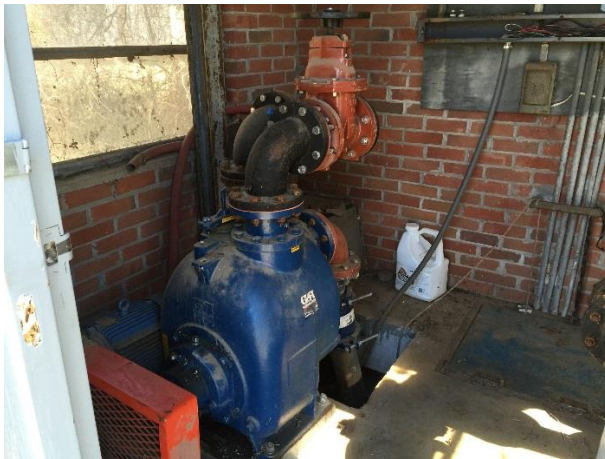
Figure 10 - Interior of Lift Sta. 2
