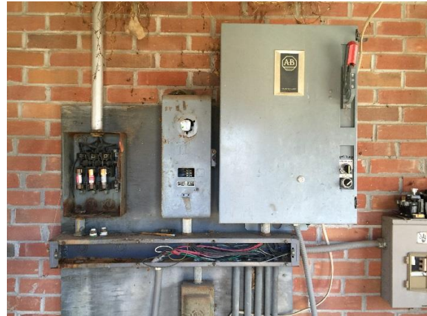
Figure 11 – Control panel at Lift Sta. 1
