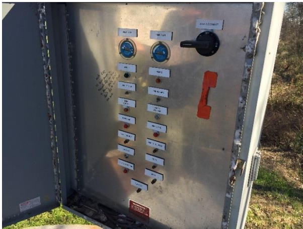
Figure 7 -Interior pump station control panel
