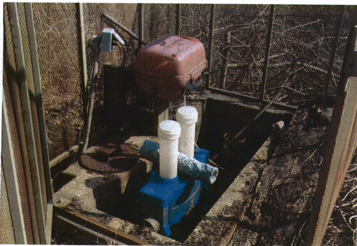
Figure 3.42 Tablet Chlorinator and Chlorine Contact Chamber
