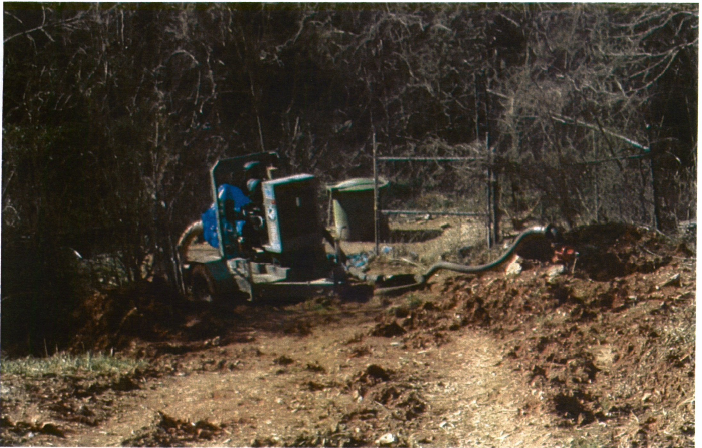
Figure 3.18 Lift Station 1 and ARWA-Installed Temporary Pump
