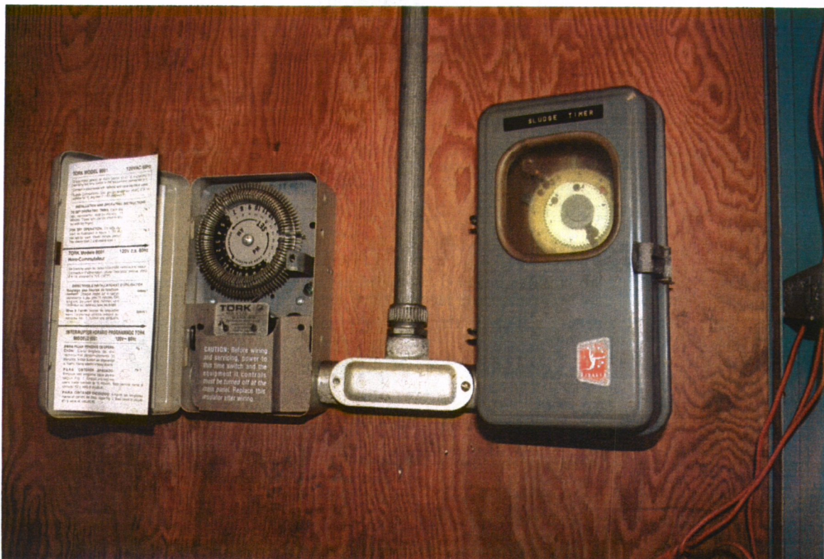
Figure 3.28 Control Panel Photo (Timers)
