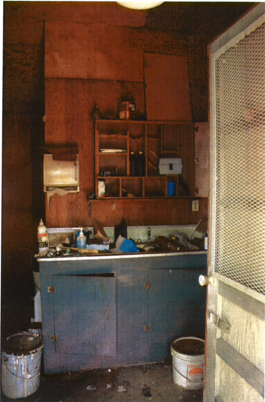
Figure 3.33 Utility Sink and Cabinet Photo
