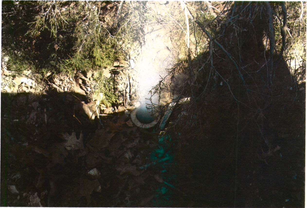
Figure 3.8 Broken Concrete Stubout
