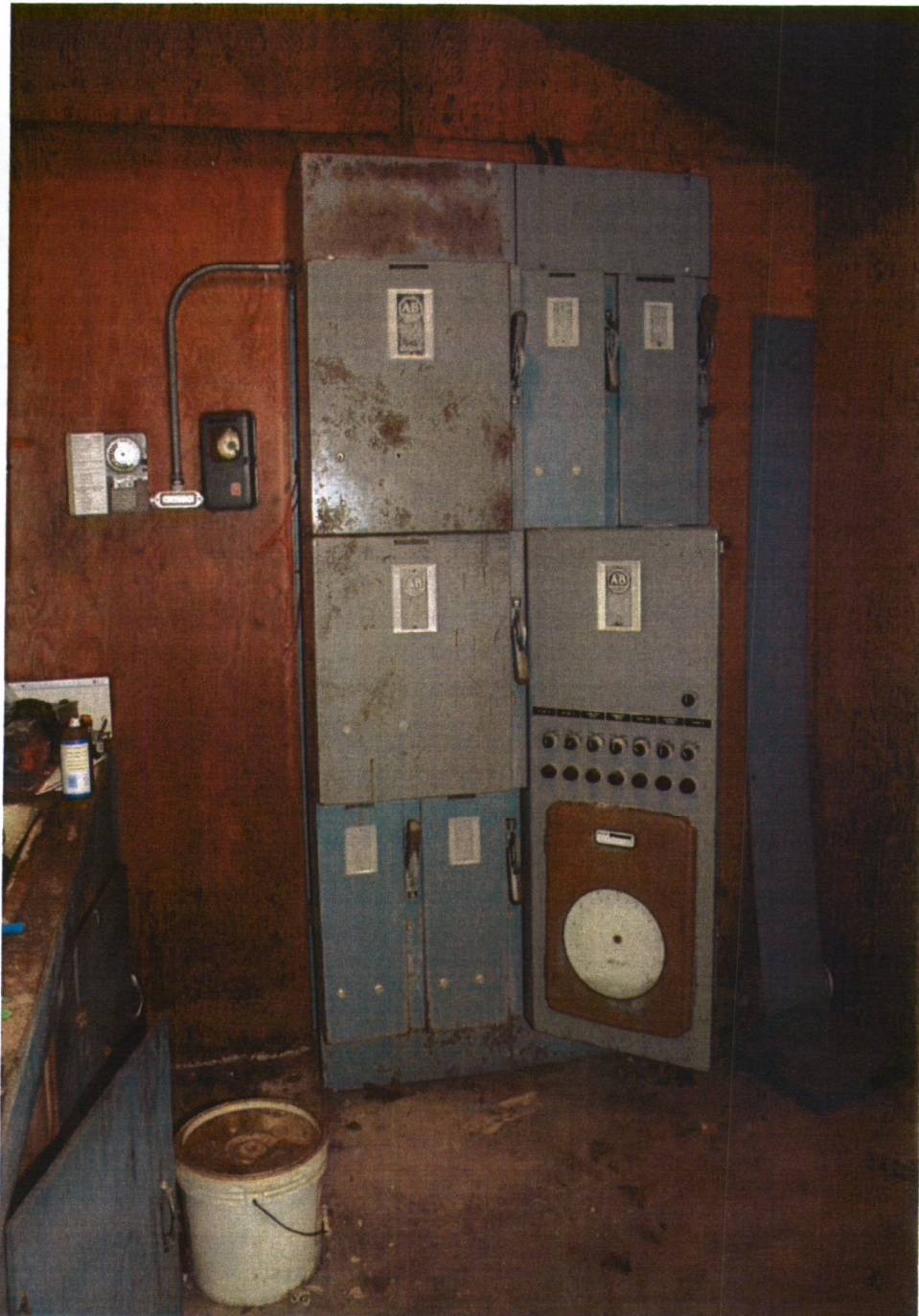
Figure 3.26 Control Panel Photo
