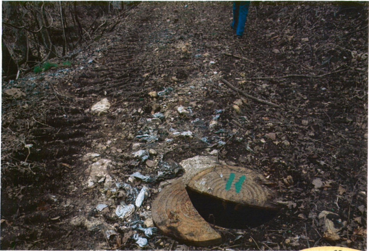
Figure 3.13 Overflow Debris Below Manhole 4-Q (ARWA MH #11)
