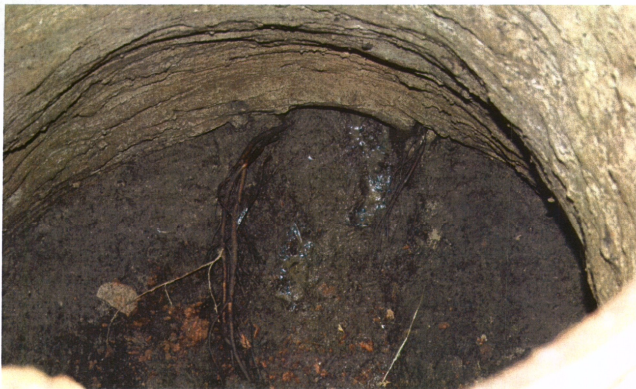
Figure 3.16 Root Intrusion in Manhole 4-N (ARWA MH #14)
