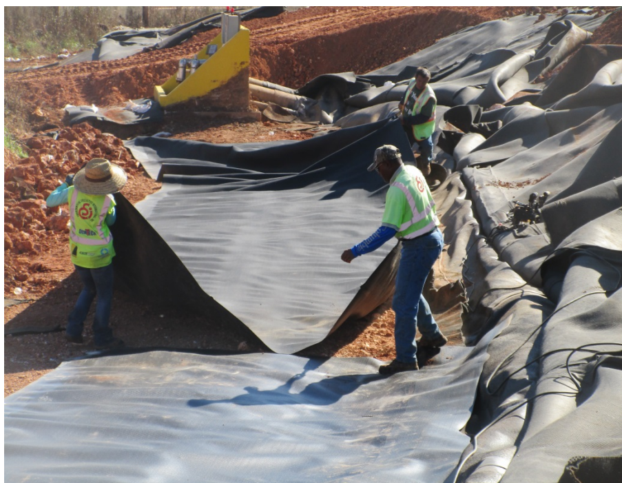
Photo 20 – Installing Rainflap at Toe of Slope before Placing Geotextile and Drainage Rock
