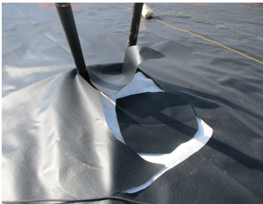
Photo 12 – Liner is cut to fit around Gas Extraction Wells, then Patch is Extrusion Welded
