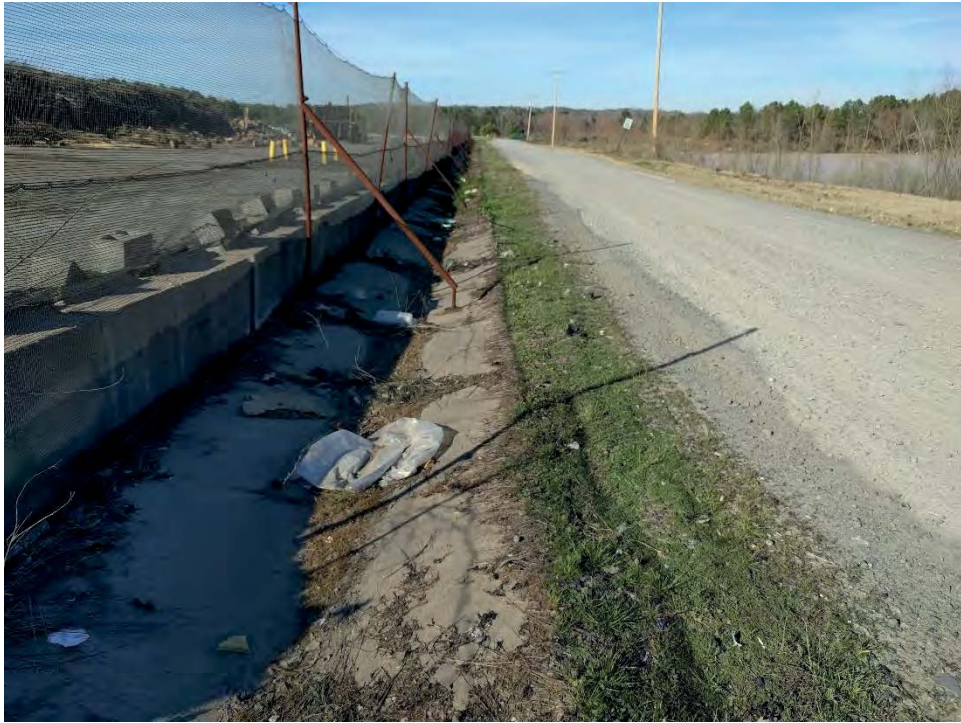
Photo 6: Litter fence and swale
