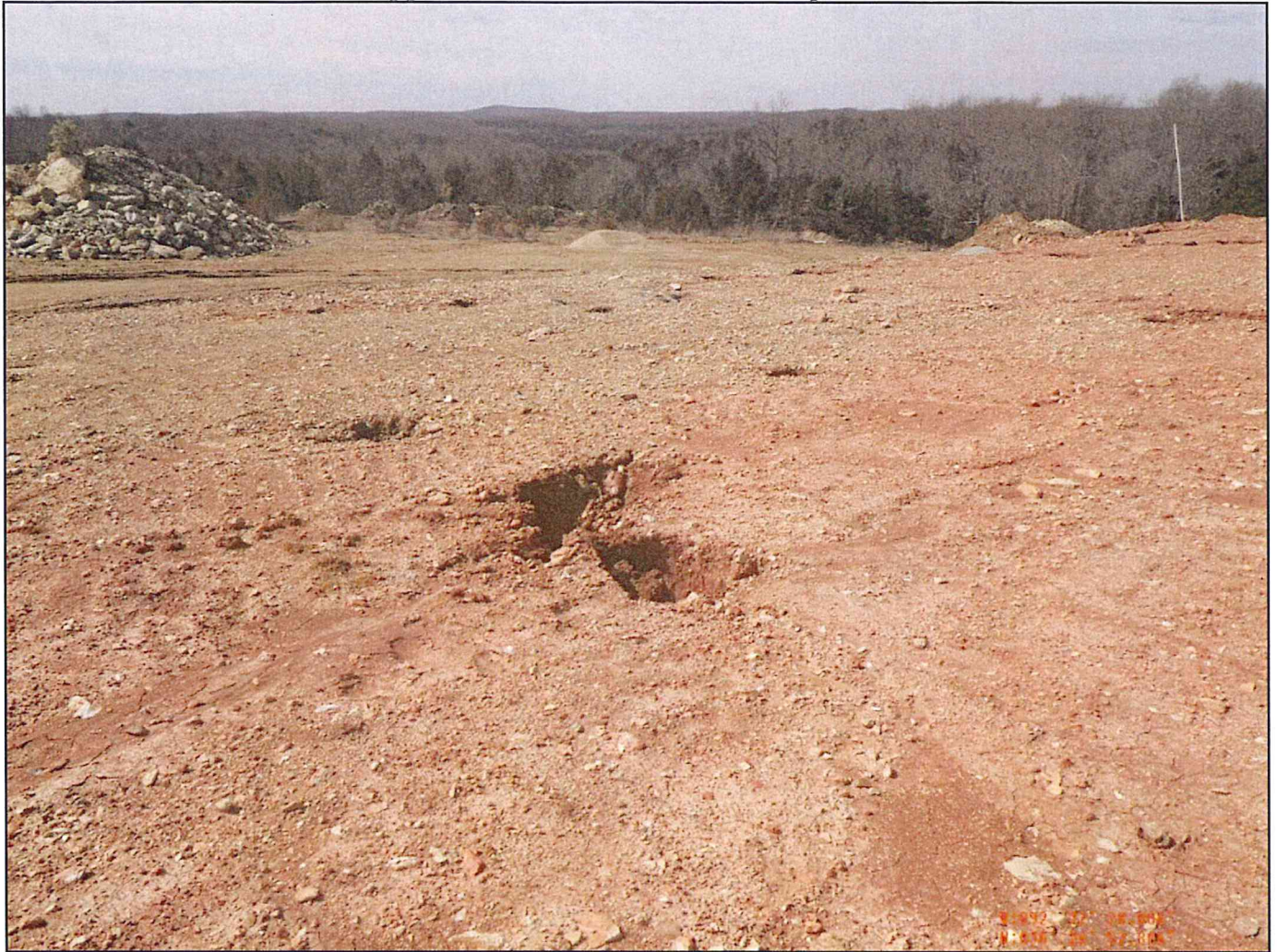
Photo #20: upper terrace soil settlement into spaces of the tires
