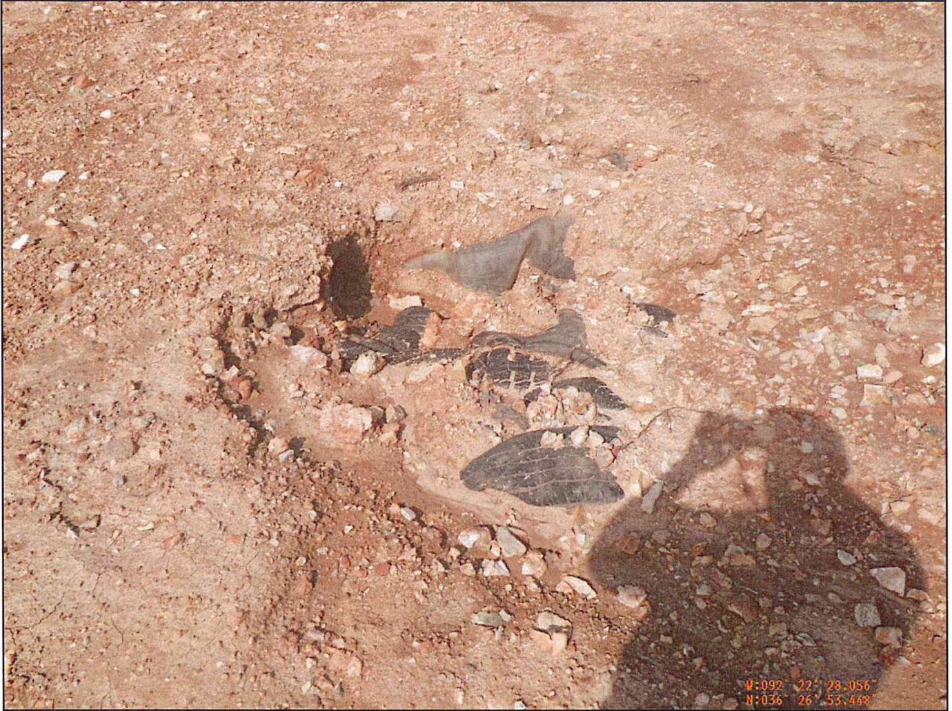
Photo #22: upper terrace soil settlement into spaces of the tires
