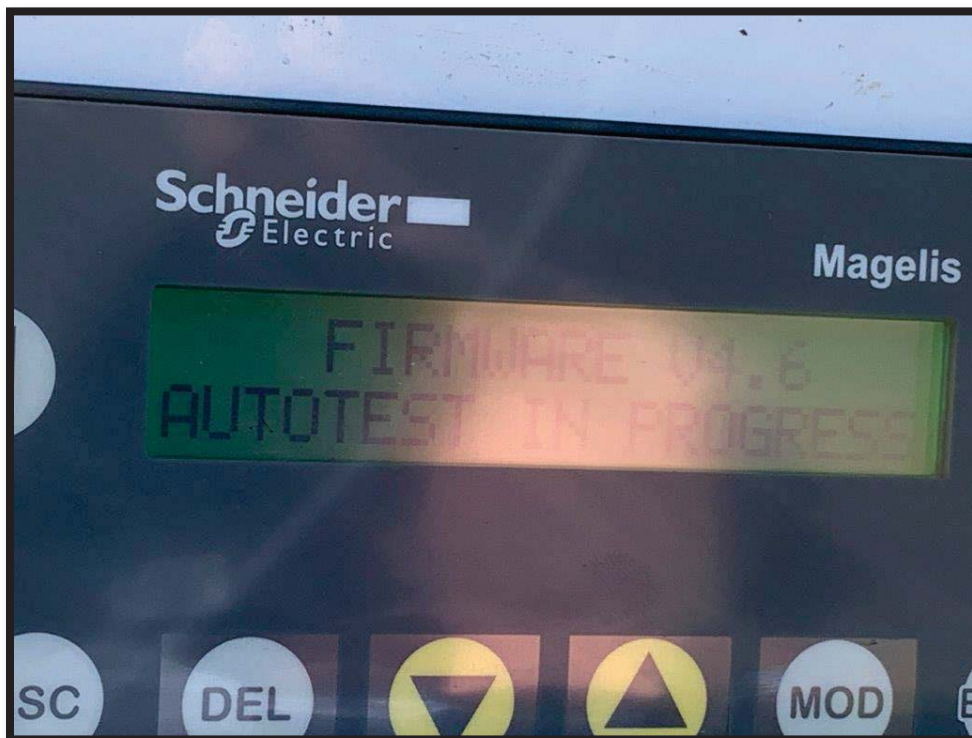
Photograph 2: View of "autotest in progress" message on panel at LCS-1.
