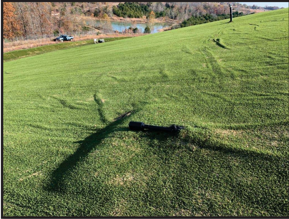
Photograph 5: View northeast of damaged vent pipe near LCS-1 (visible in distance).
