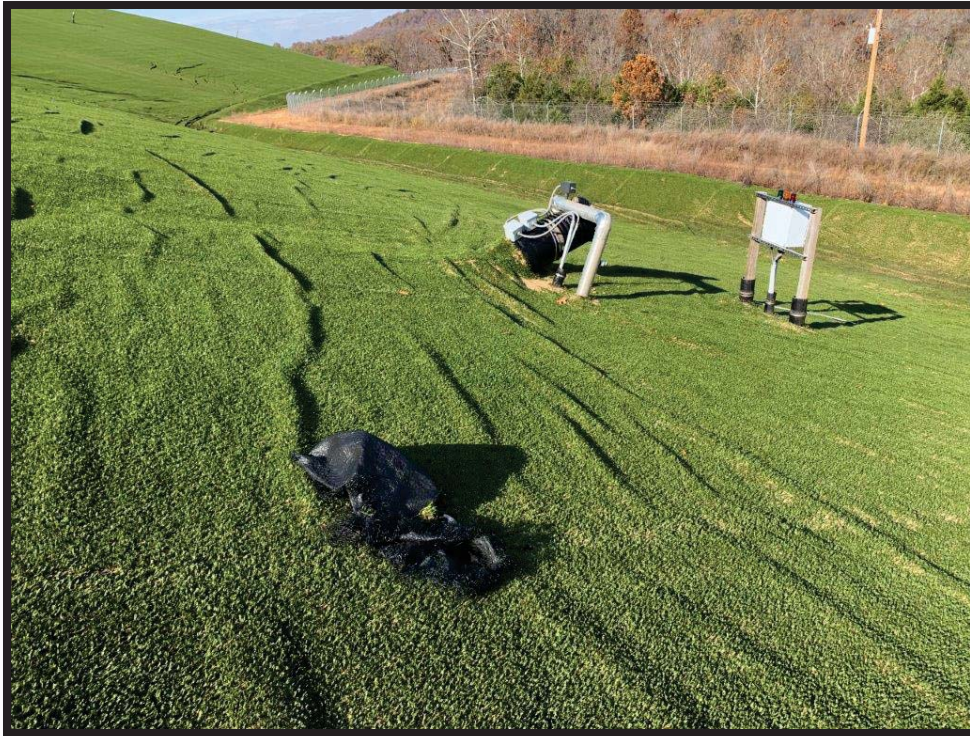
Photograph 3: View west of torn liner piece near LCS-1.
