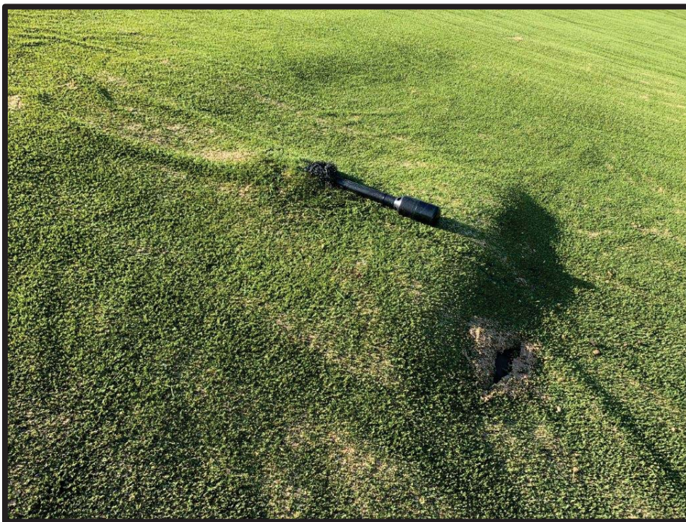
Photograph 4: View southwest of damaged vent pipe near LCS-1.
