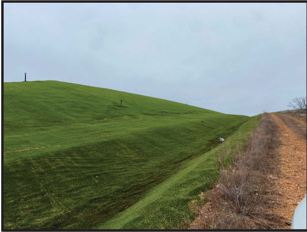
Photograph 5: View of damages turbine vent near LCS-6
