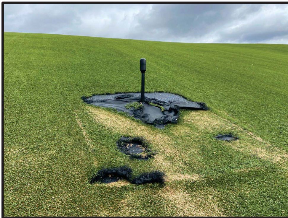
Photograph 4: View of damaged closure turf near LCS-4.
