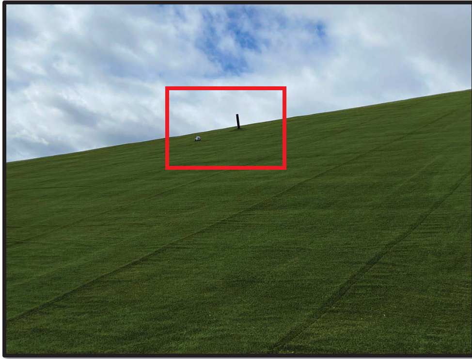
Photograph 5: View of detached turbine vent near LCS-8.
