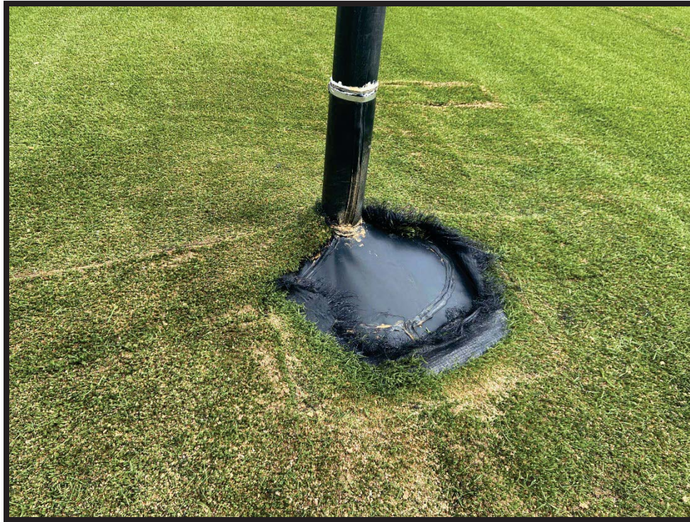
Photograph 3: View of damaged closure turf near LCS-4.
