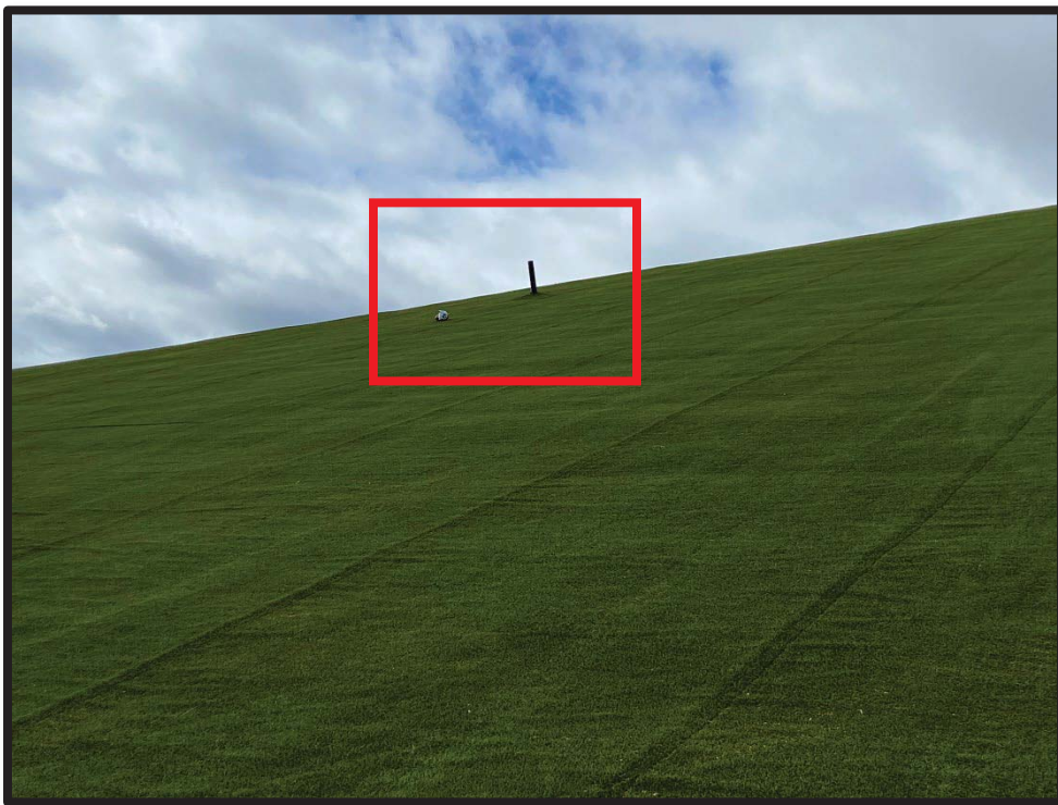
Photograph 4: View of detached turbine vent near LCS-8.
