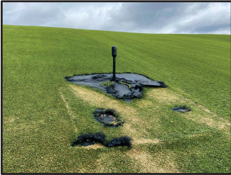
Photograph 3: View of damaged closure turf near LCS-4.
