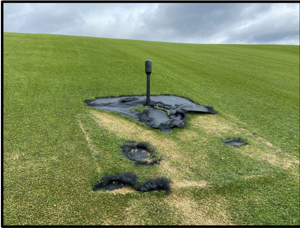
Photograph 3: View of damaged closure turf near LCS-4.
