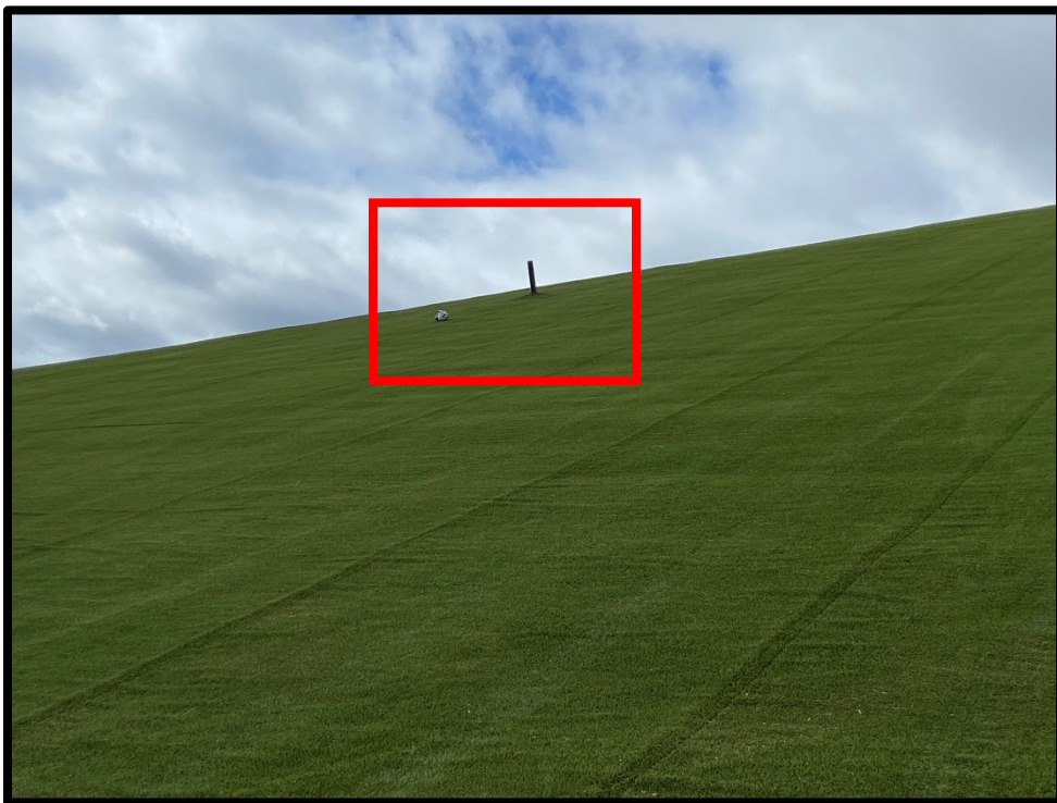
Photograph 4: View of detached turbine vent near LCS-8.
