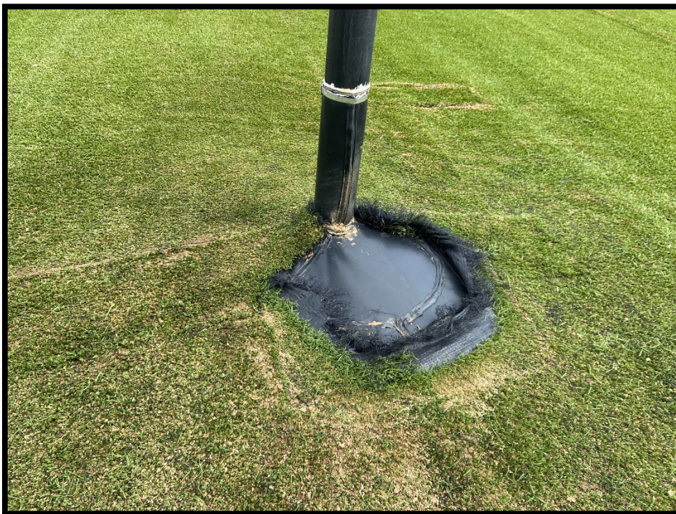
Photograph 2: View of damaged closure turf near LCS-4.
