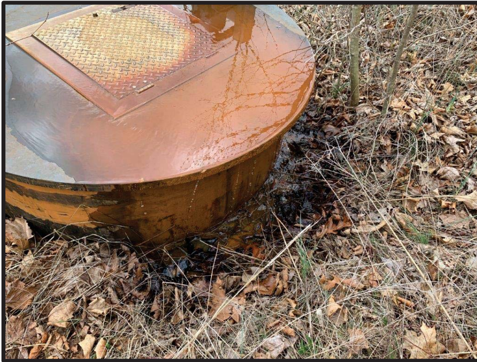
Photograph 3: View of VLCS-1 at full capacity and overflowing.
