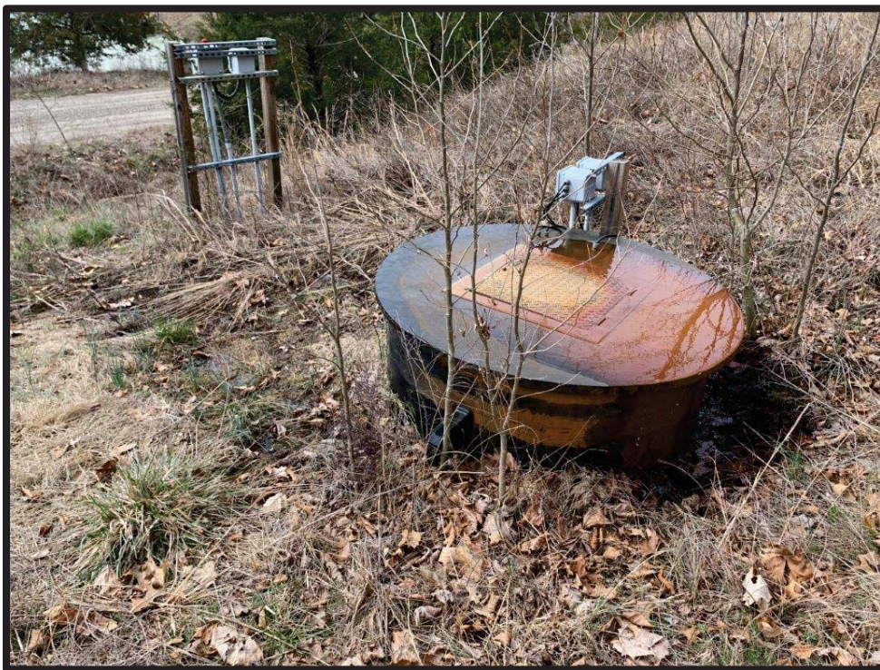
Photograph 4: Additional view of VLCS-1 at full capacity and overflowing.
