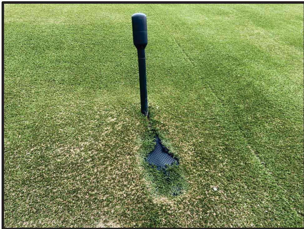
Photograph 10: Torn closure turf around PRV on south side of Area 1-3.
