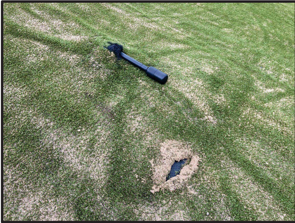
Photograph 5: Broken PRV and closure turf tear on the north side of Area 1-2, near LCS-1.
