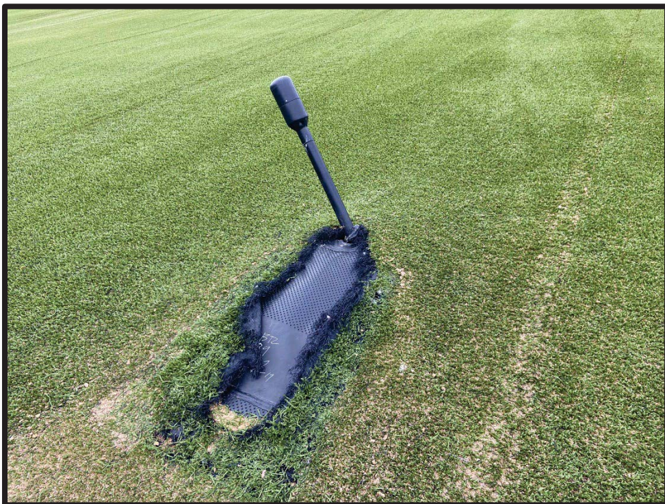
Photograph 6: Bent PRV and closure turf tear on north side of Area 1-2, near LCS-1.
