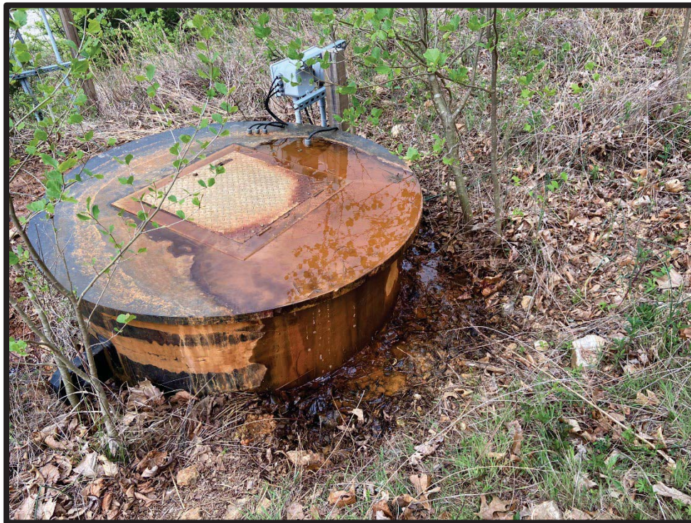
Photograph 2: View of VLCS-1 at full capacity and overflowing.
