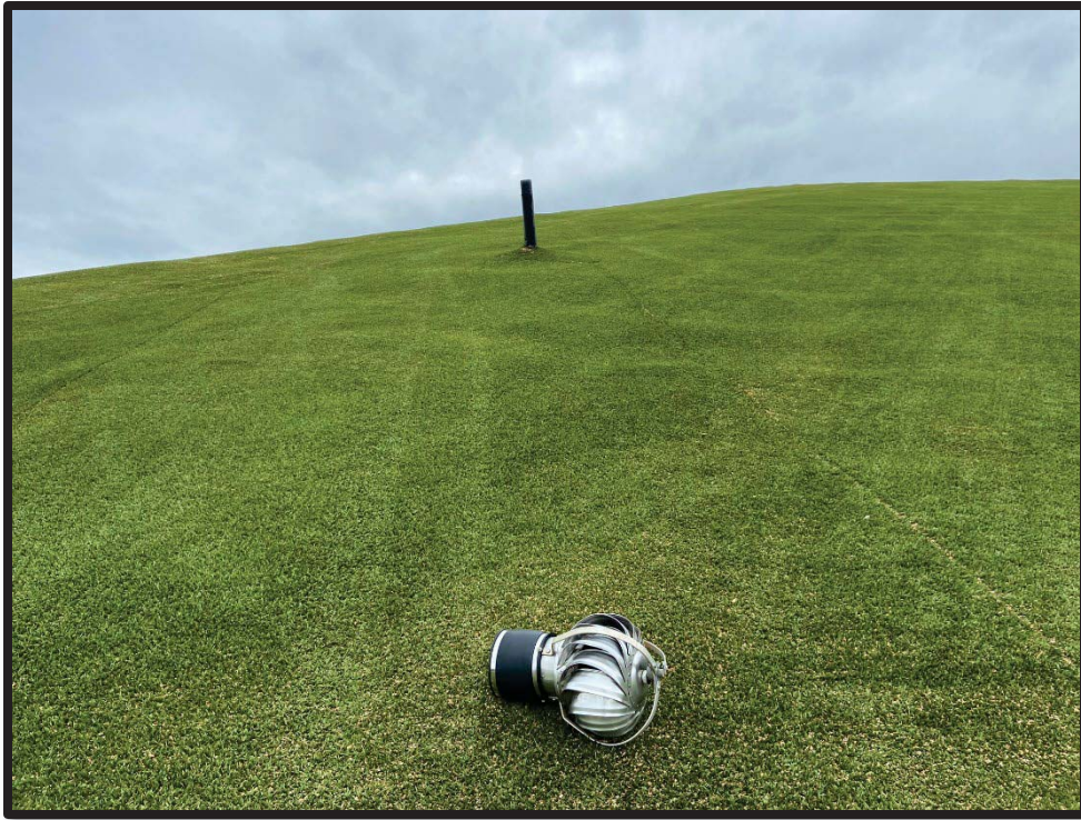
Photograph 11: Damaged turbine vent on Area 1-3, near LCS-8.
