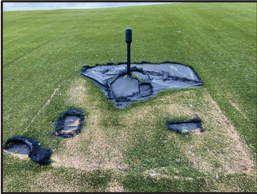
Photograph 7: Torn closure turf on south side of Area 1-2, near LCS-4.
