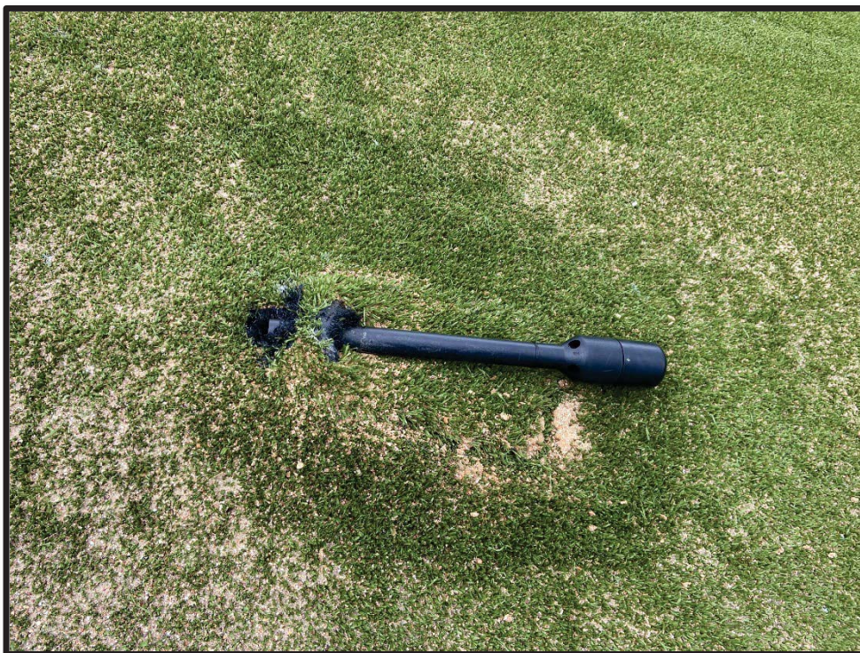
Photograph 4: Broken PRV on the east side of Area 1-2.
