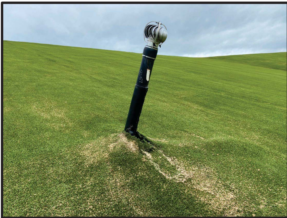
Photograph 12: Torn closure turf around turbine vent on Area 1-3, near LCS-7.
