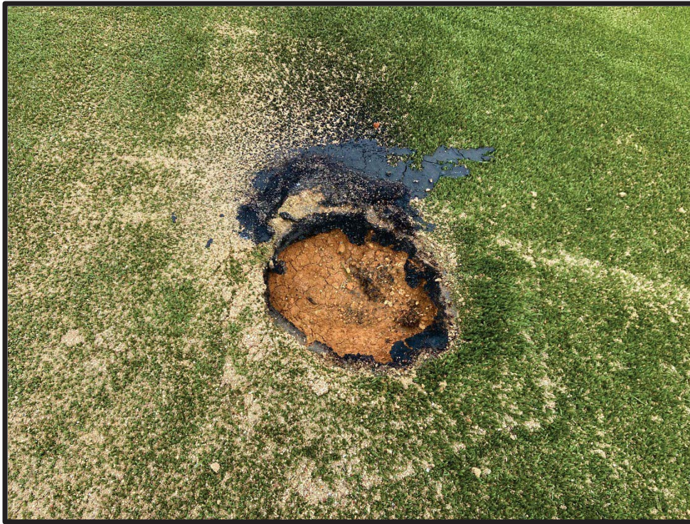
Photograph 13: Torn closure turf where vent was on Area 1-3, near LCS-6.
