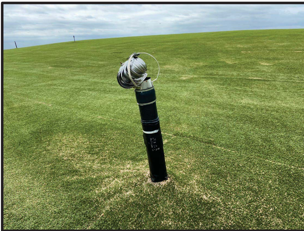
Photograph 14: Damaged turbine vent atop Area 1-3.
