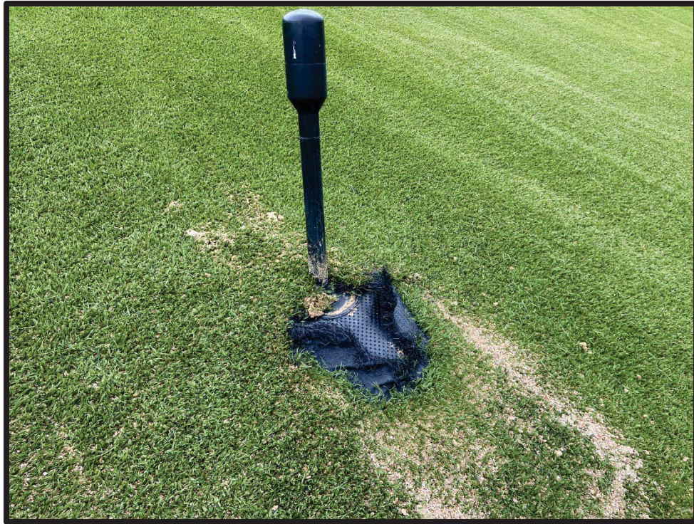
Photograph 9: Closure turf tear around PRV on Area 1-2, near LCS-4.
