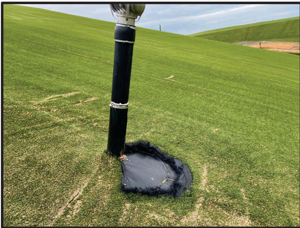
Photograph 8: Torn closure turf on south side of Area 1-2, near LCS-4.
