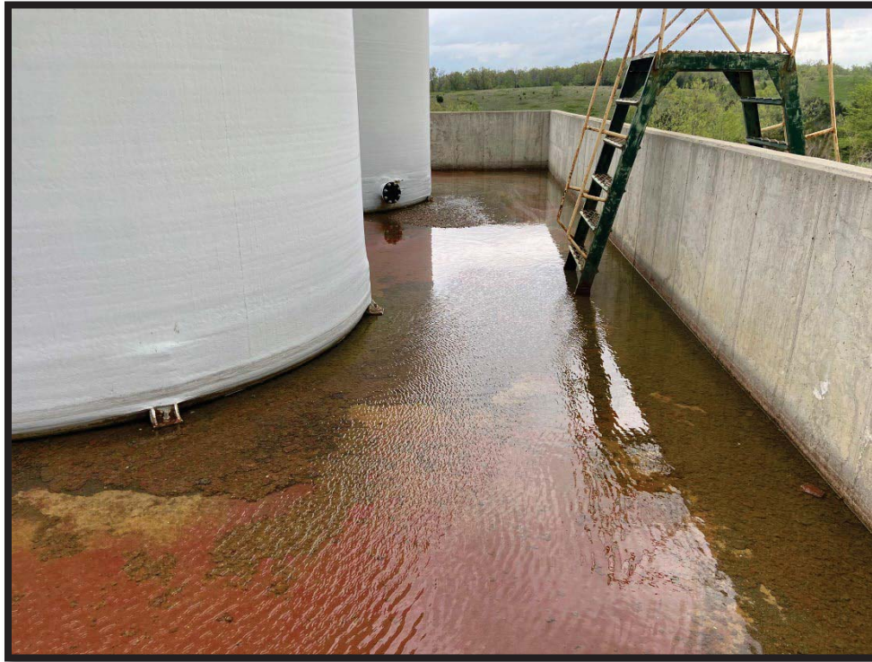
Photograph 1: View of stormwater in leachate tank containment.
