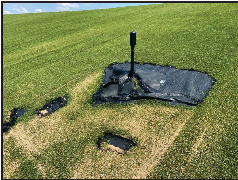
Photograph 4: Closure turf tear around PRV on the south side of Area 1-2, near LCS-4.
