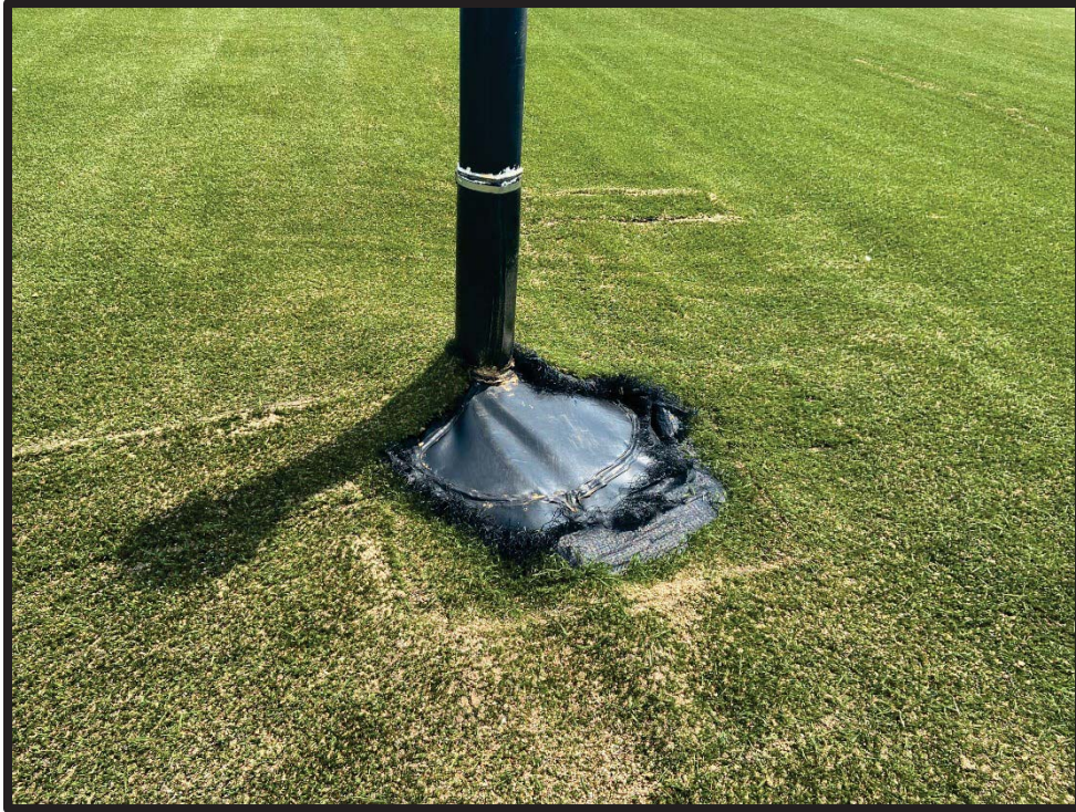
Photograph 3: Closure turf tear around turbine vent on the south side of Area 1-2, near LCS-4.
