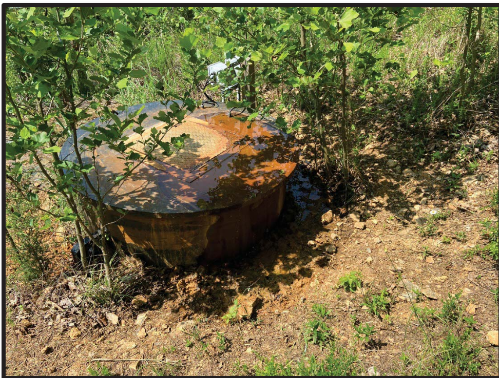
Photograph 2: View of overflow at VLCS-1.
