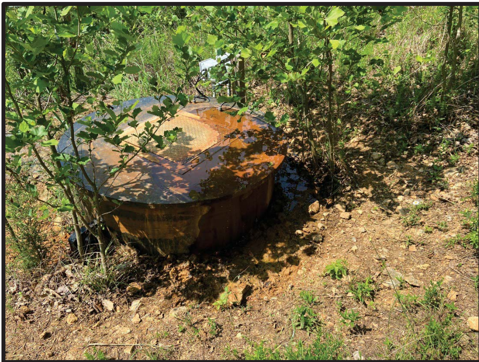
Photograph 2: View of overflow at VLCS-1.
