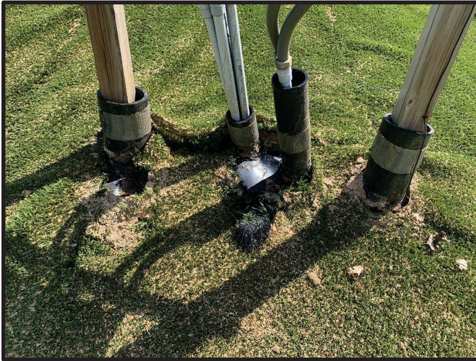
Photograph 7: Closure turf damage at base of LCS-4.
