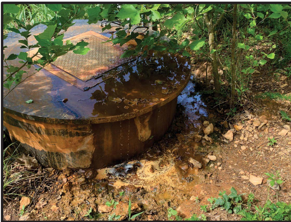
Photograph 6: View of overflow at VLCS-1.
