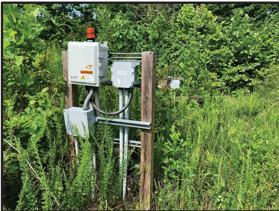
Photograph 4: View southwest of VLCS-2 control panel and overgrown vegetation.
