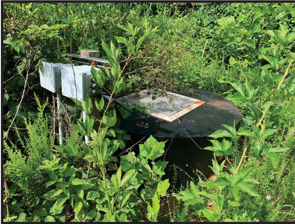
Photograph 3: View southwest of VLCS-2 sump overgrown with vegetation.
