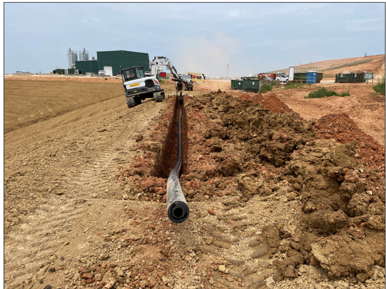
Photo No. 5 Contractor installing 3"x6" HDPE dual contained leachate forcemain on the east perimeter of Cell 8.
