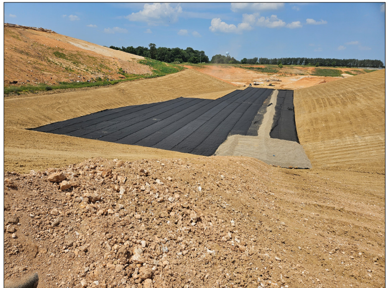
Photo No. 11 Looking west at Geocomposite installed on the cell floor and completed leachate collection corridor
