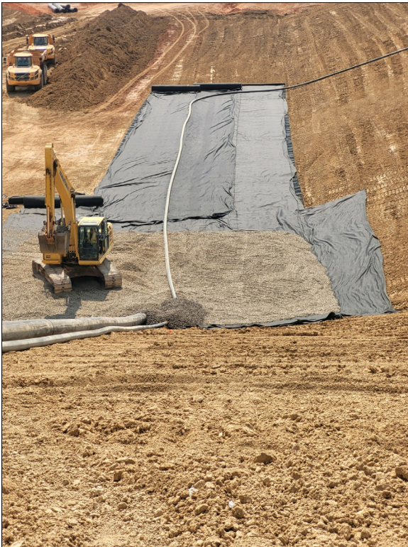
Photo No. 9 Contractor installing aggregate in leachate sump along with 6" HDPE cleanout pipe.
