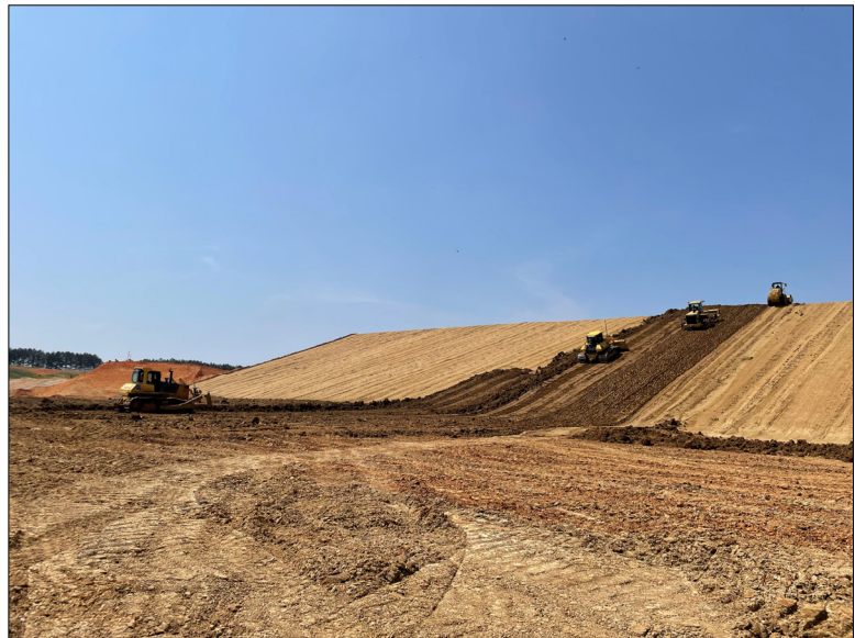
Photo No. 2 Contractor processing, spreading and compacting clay liner on north slope.
