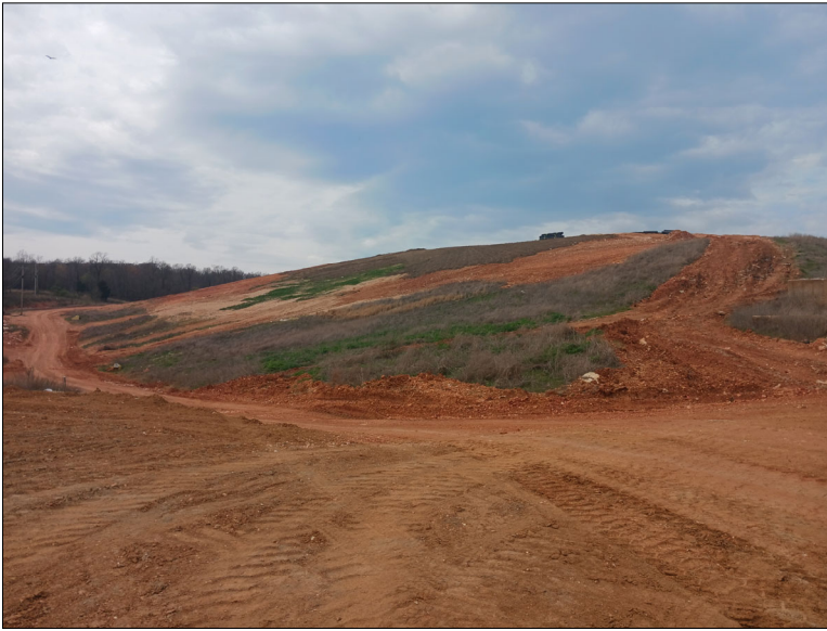
Photo No. 4 Looking west at the south slope of the Class 4 Landfill.
