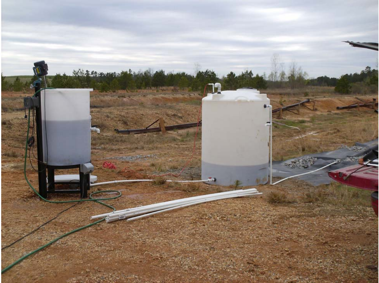
Figure 5.2. Pilot-scale treatment system installed on the Reynolds site.
