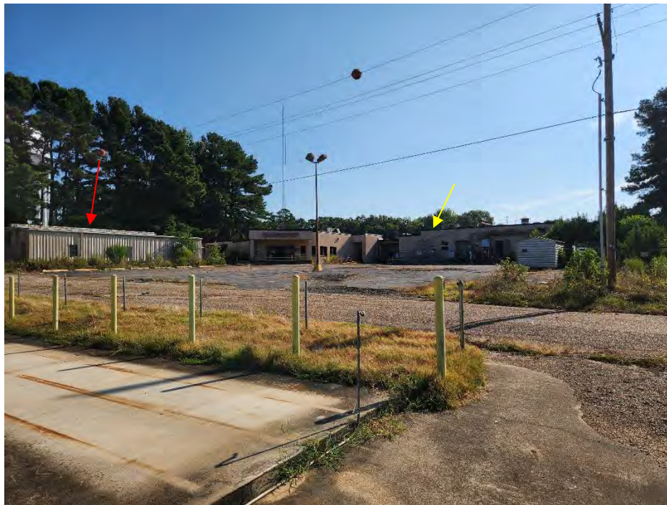
Photo 10: This photograph shows a view of assumed ACM roofing material on the Purchasing Department building (red arrow) and the Hospital Building (yellow arrow).
