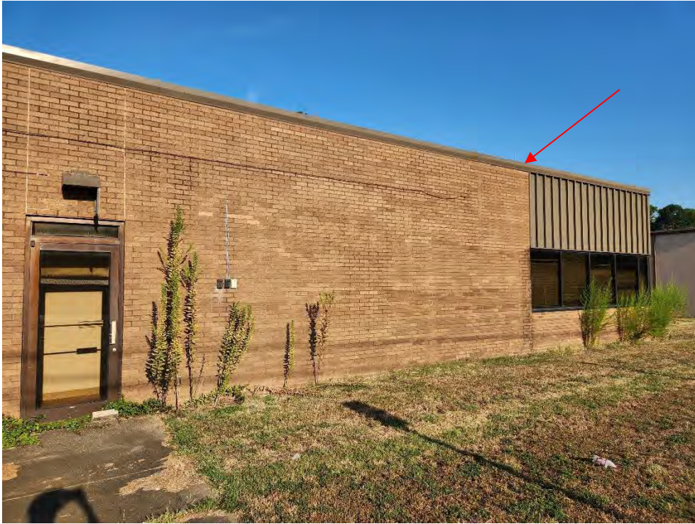
Photo 11: This photograph shows a view of assumed ACM roofing material on the Medical Plaza building (red arrow).
