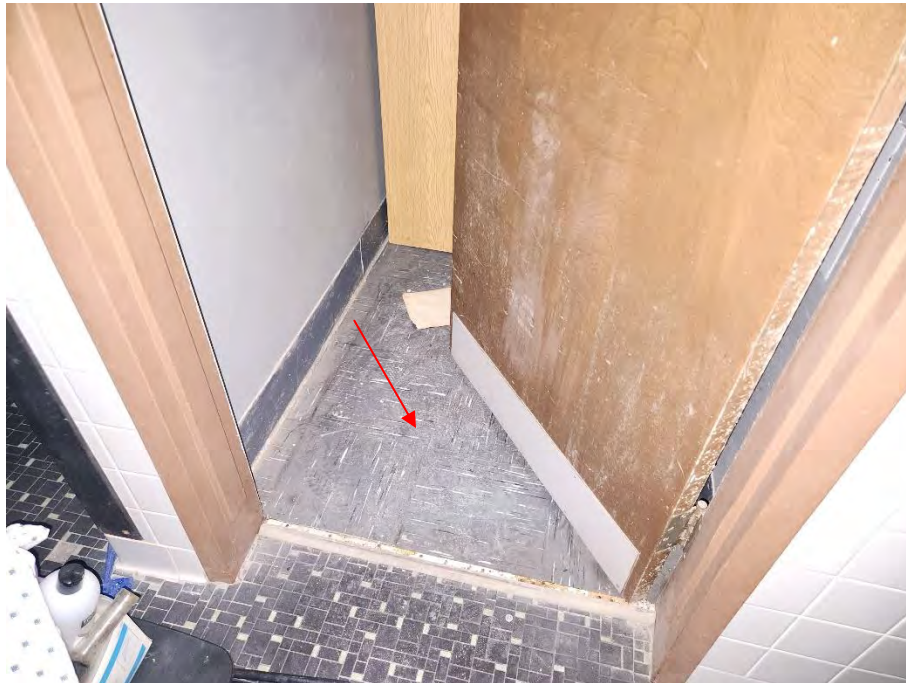
Photo 7: This photograph shows ACM 12- by 12-inch gray with white and black streaks and black mastic (HS-VFT07) in the operating room doctor's lounge of the Hospital building (red arrow).
