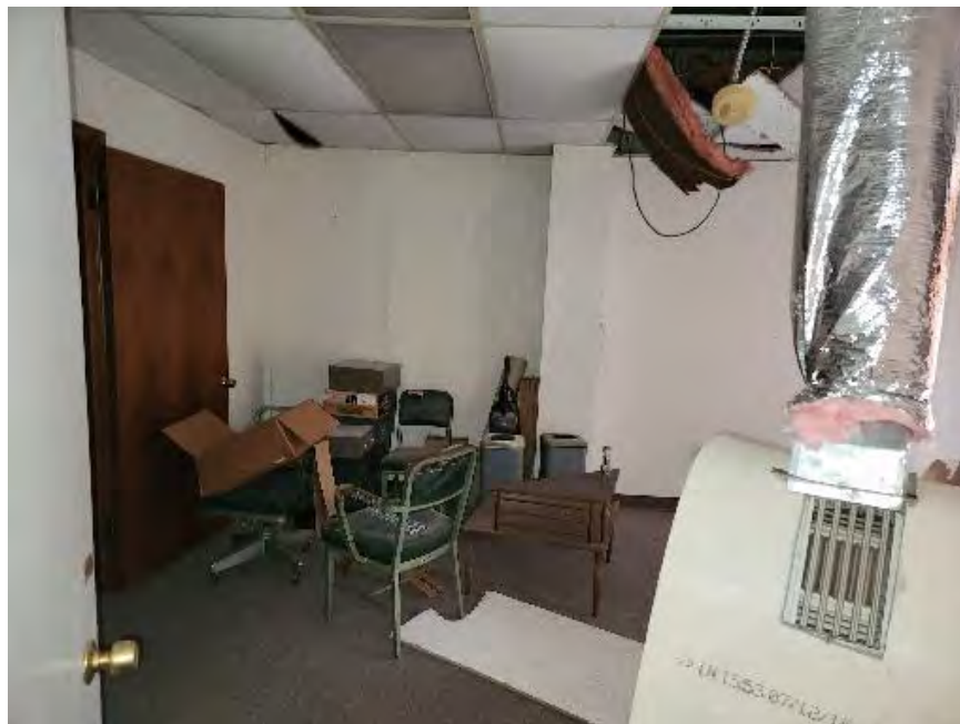
Photograph 12 (Overview): View of office space in the southwest corner of the Medical Arts building. Heating, ventilation, and air conditioning (HVAC) ducting was observed falling down from the ceiling.
