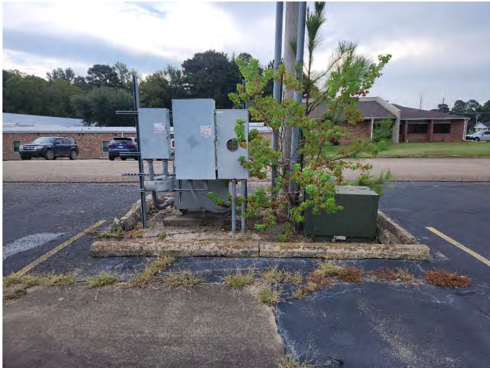
Photograph 48 (East): View of a pad-mounted transformer on the eastern side of the subject property.
