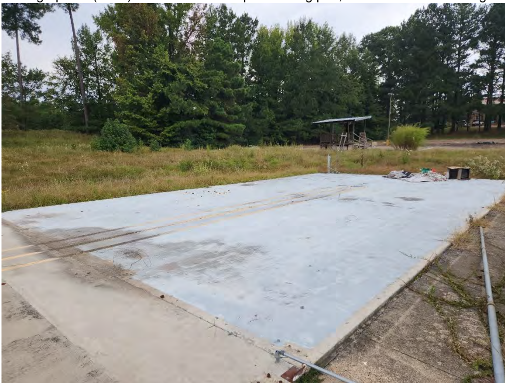
Photograph 30 (Northwest): View of the former helicopter hangar concrete foundation with some general refuse.
