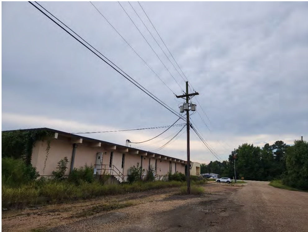
Photograph 45 (North): View of pole-mounted transformers behind the Medical Clinics building.
