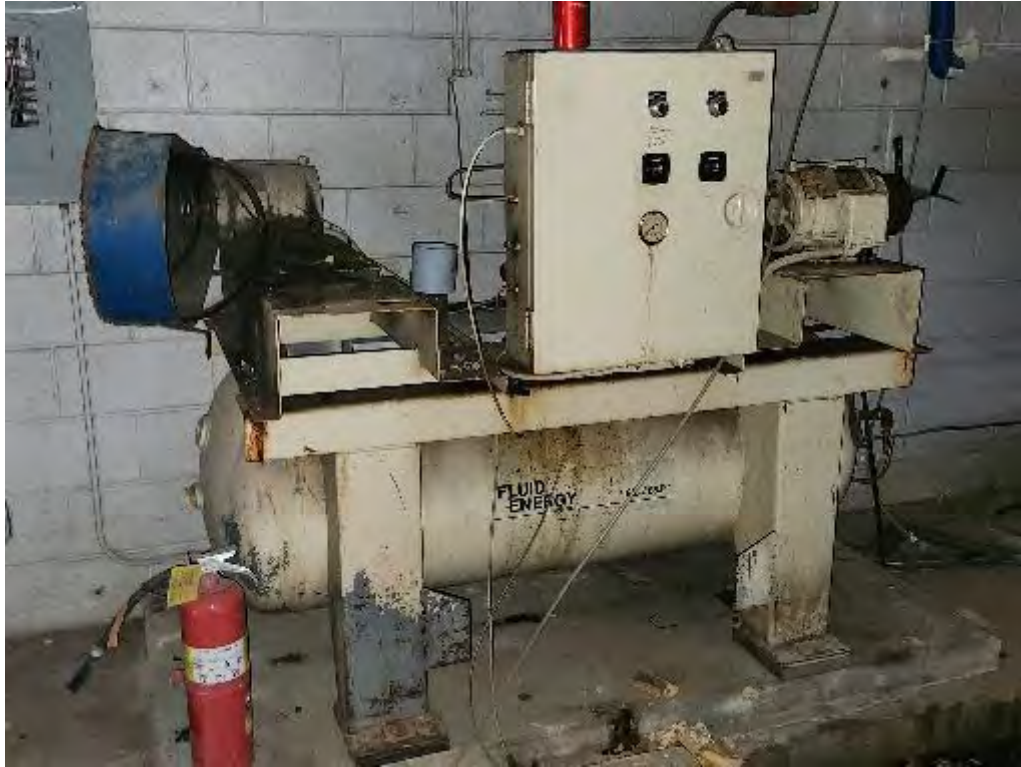
Photograph 21 (NA): View of an air compressor in the boiler room of the main Hospital building.
