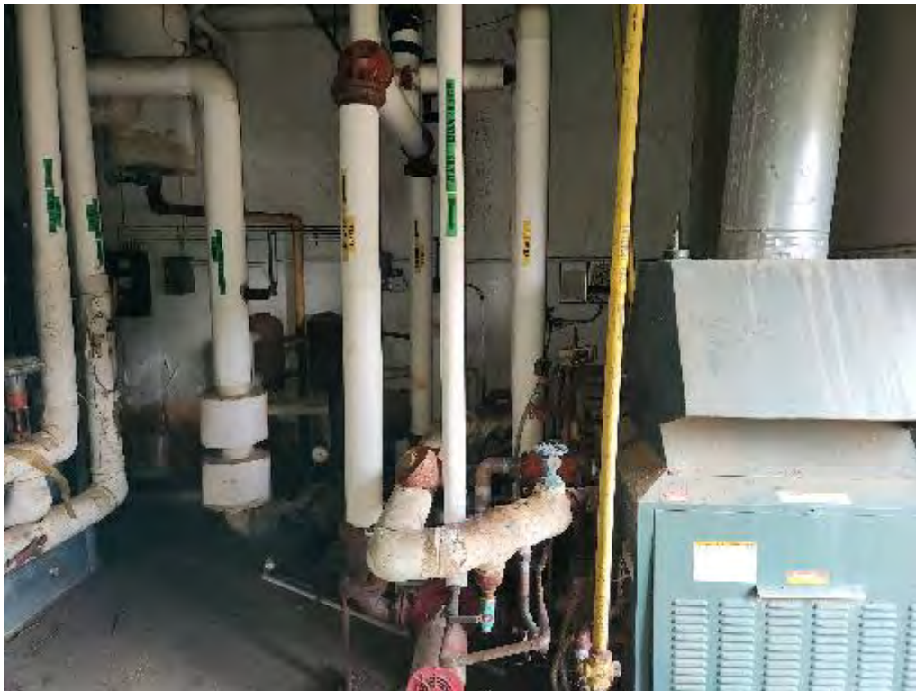
Photograph 32 (North): View of piping throughout the utility room on the east side of the main Hospital building.
