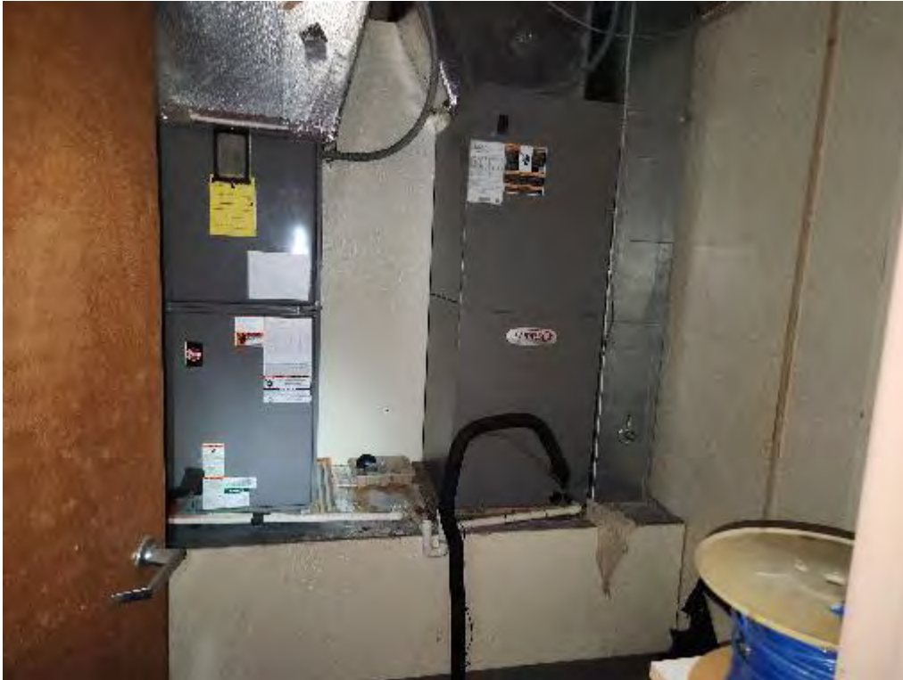
Photograph 9 (Overview): View of heating ventilation and air conditioning (HVAC) system in the subject property building.
