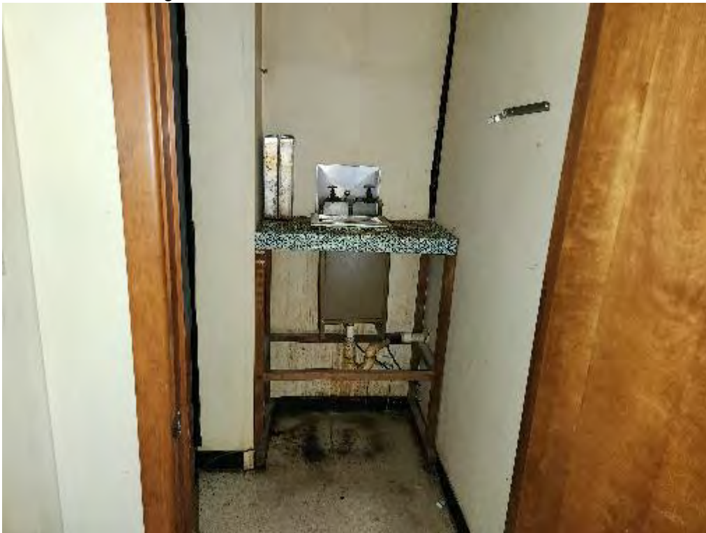
Photograph 6 (Overview): View of former dark room in the back northwest corner of the Medical Arts building. Staining was observed on the floor beneath the sink. The sink drains to the sewer system.
