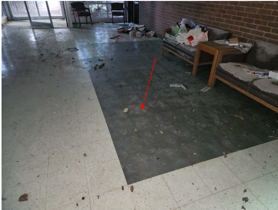
Photo 5: This photograph shows ACM 12- x 12-inch gray vinyl floor tile and black mastic (HS-VFT04) in the front entryway of the Hospital building (red arrow).
