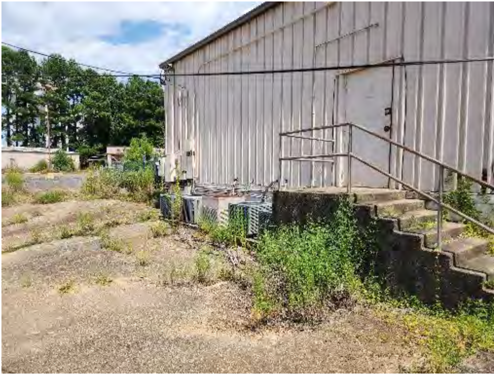
Photograph 13 (Northeast): View of the back of the Medical Arts building (west side). Air conditioning units and electrical paneling is visible.
