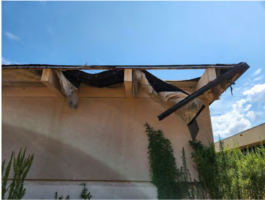
Photo 7: This photograph shows a closeup view of the assumed ACM roofing material on the Medical Clinics building and its damage.
