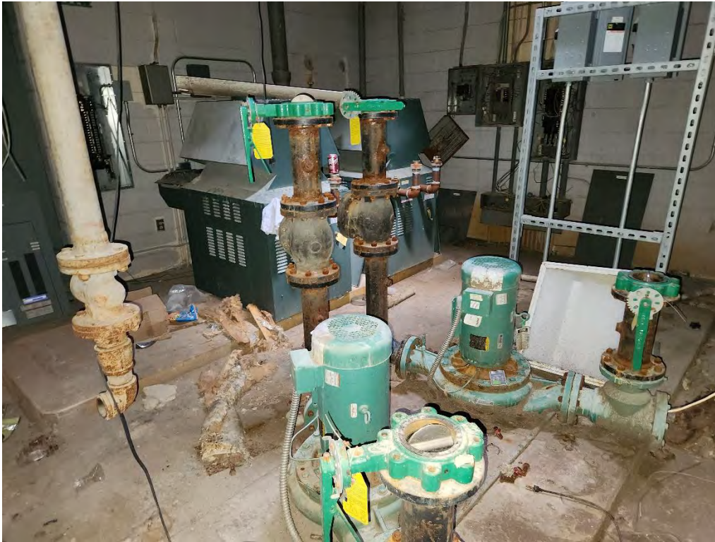
Photograph 17 (Northeast): View of north side of the boiler room in the Hospital building.
