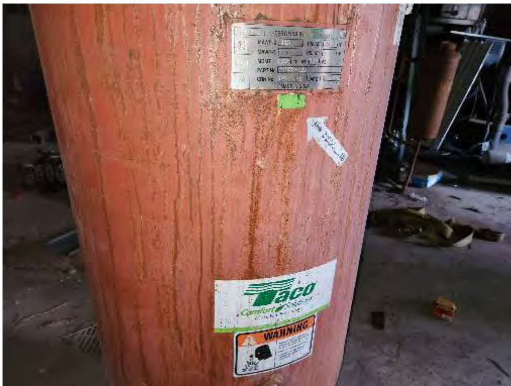
Photograph 18 (NA): View of label on the pressure tank in Photograph 17 in the boiler room of the main Hospital building.
