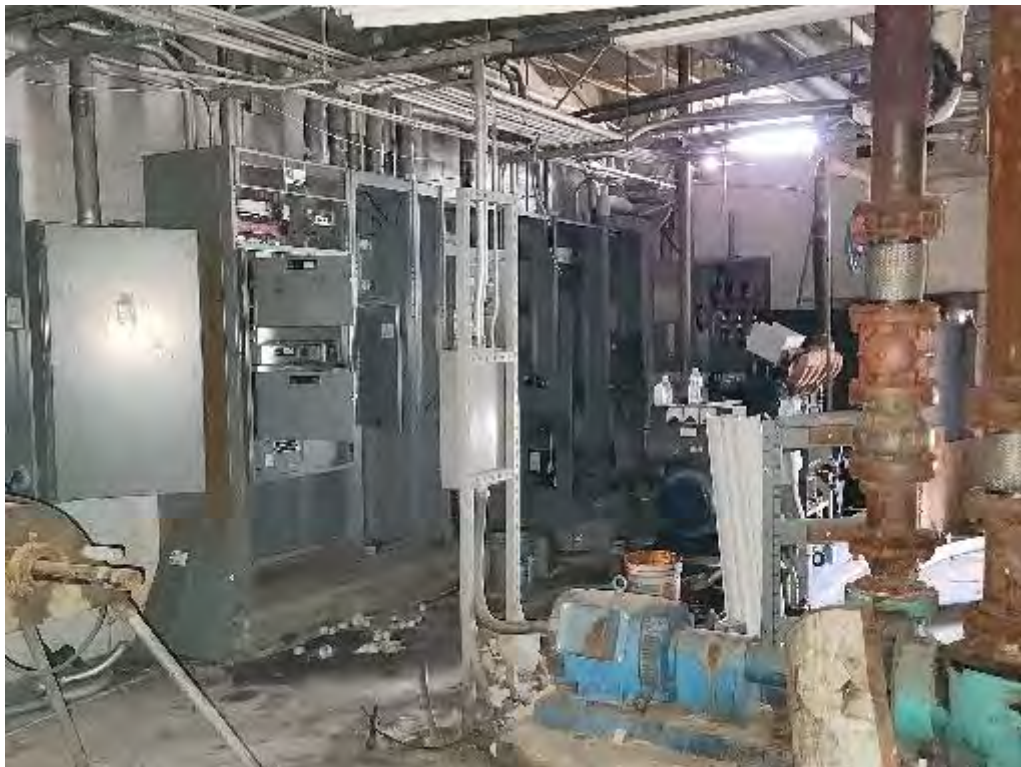
Photograph 24 (Southwest): View of electrical paneling within the boiler room in the main Hospital building.
