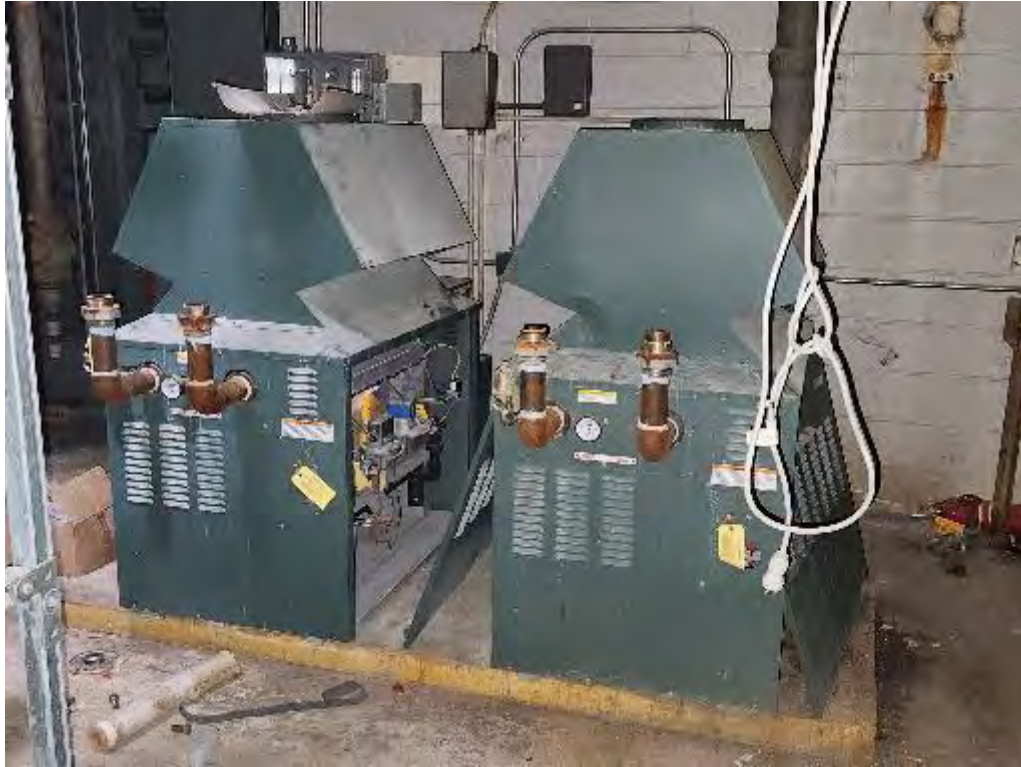
Photograph 25 (West): View of boilers in the boiler room of the Hospital building.
