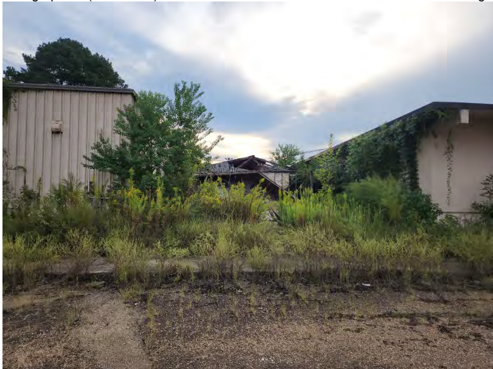
Photograph 44 (East): View of the collapsed wooden structure between the Medical Arts and Medical Clinics building.
