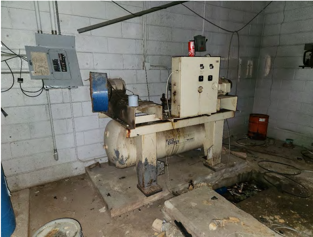
Photograph 13 (Southeast): View of the air compressor in the boiler room of the Hospital building, with staining on the floor.
