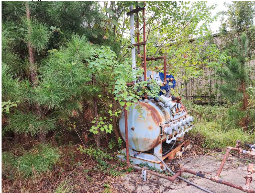
Photograph 20 (Southeast): View of generator in the fenced area of the subject property.
