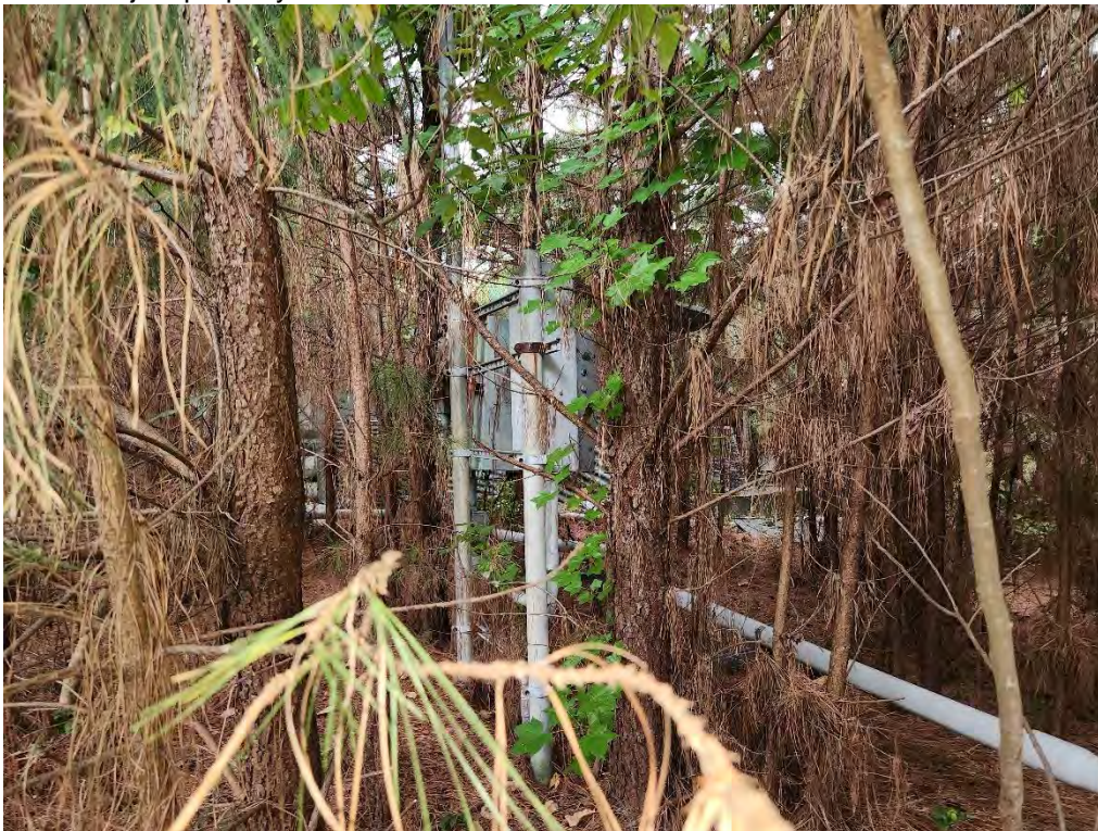
Photograph 22 (South): View of the transformer in the fence area of the subject property, obscured by the dense vegetation.
