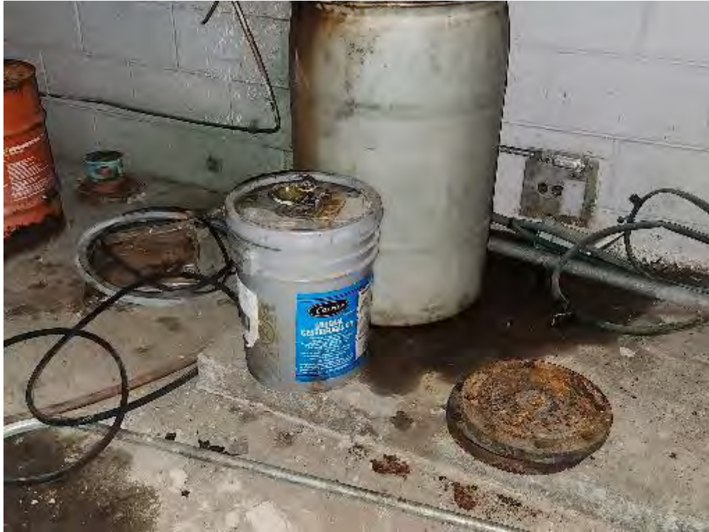
Photograph 23 (NA): View of an unlabeled 55-gallon drum and 5-gallon bucket of mineral oil with heavy staining surrounding them (in the boiler room).
