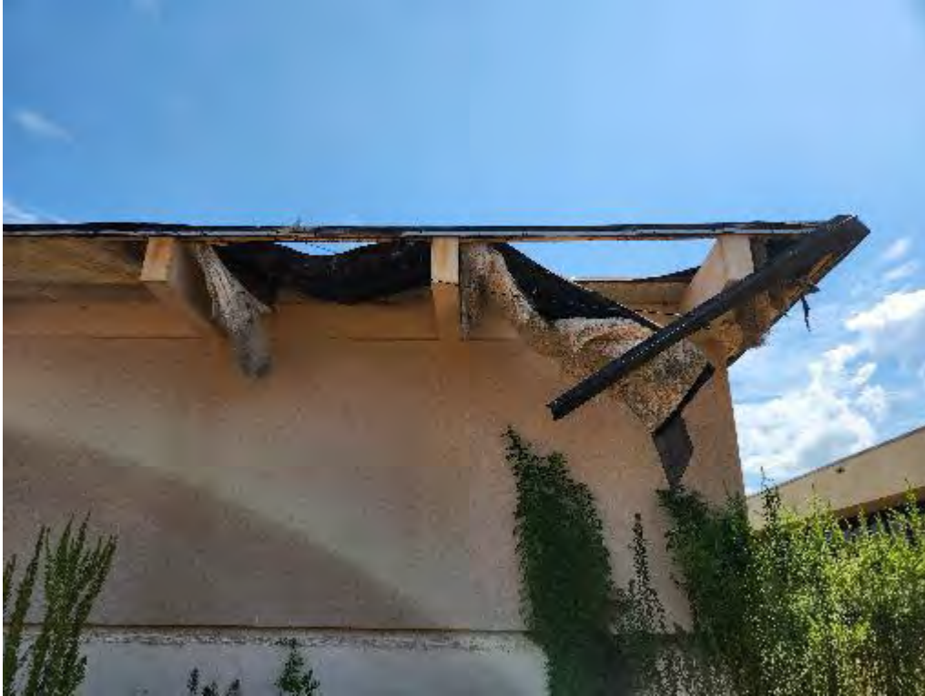
Photograph 27 (East): View of leaking roof edge along the back southwest corner of the Medical Clinics building.
