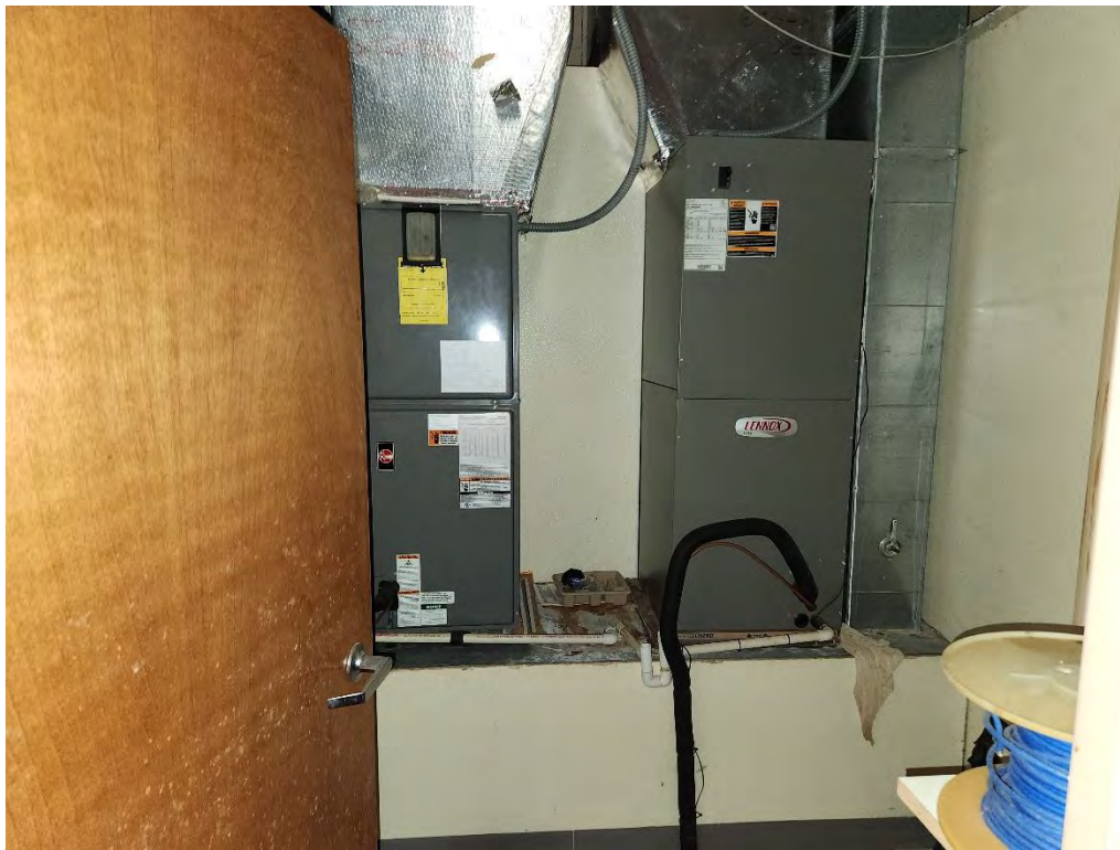
Photograph 25 (South): View of the heating, ventilation, and air conditioning (HVAC) system in the EMS building.
