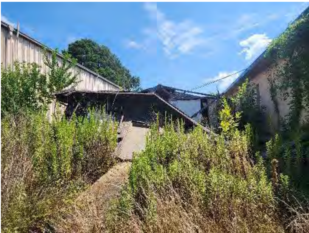
Photograph 16 (East): Back view of collapsed wooden structure between the two clinic buildings. The structure was unsafe for entry.
