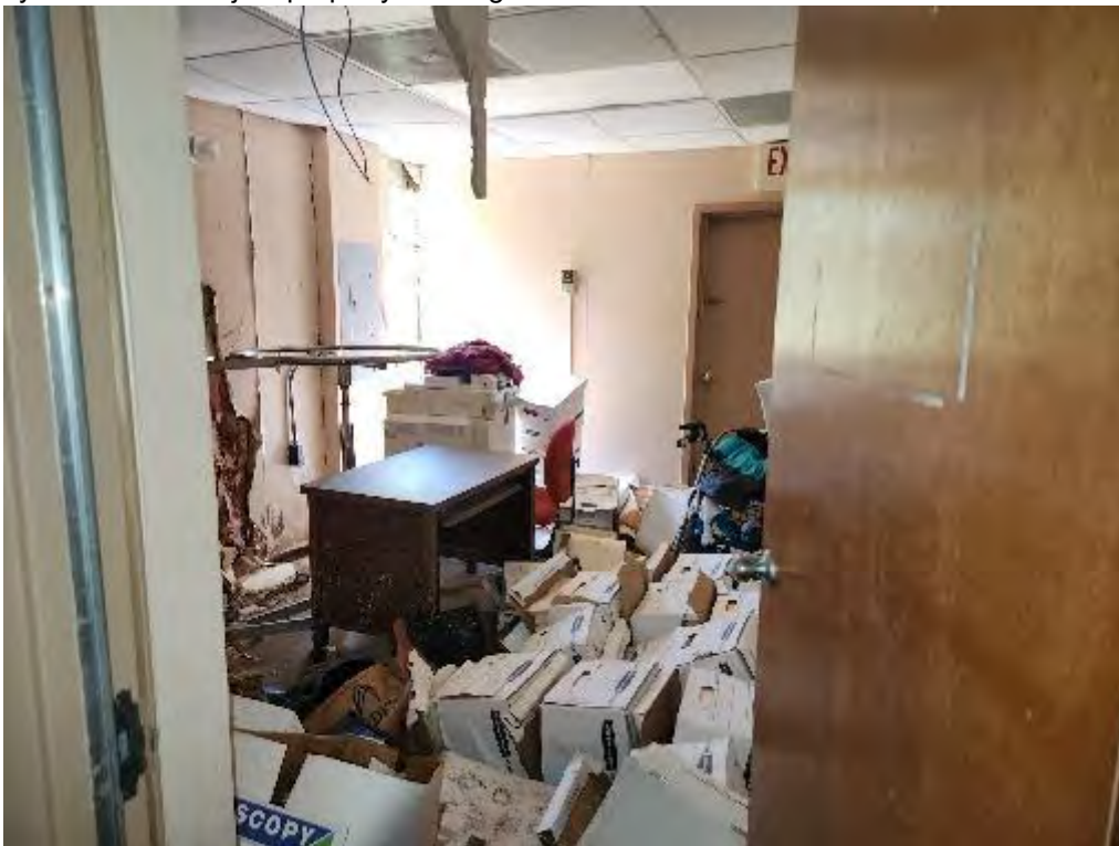
Photograph 10 (West): View of back room with files along the west side of the subject property building. A hole is along the back wall of the room and signs of water damage are evident.
