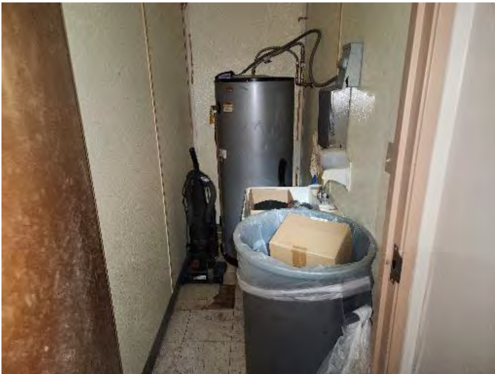
Photograph 4 (Overview): View of water heater in a closet on the east side of the subject property building.
