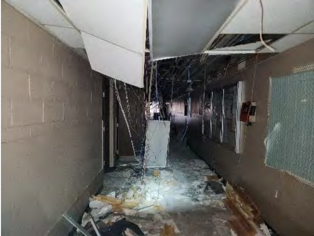
Photograph 7 (West): View of hallway off the main entranceway of the Hospital building with various electronic wires hanging from the ceiling.
