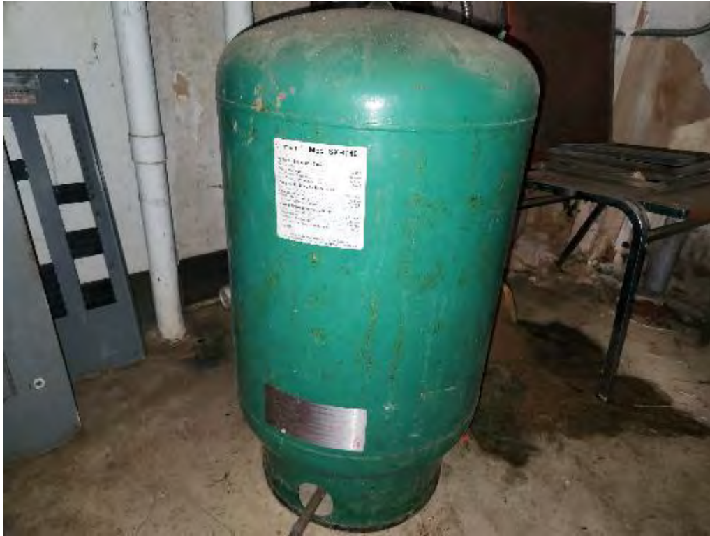
Photograph 31 (NA): View of Hydronic expansion tank within the utility room on the east side of the main Hospital building.
