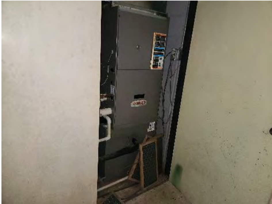
Photograph 19 (Overview): View of the heating and air condition system within the Medical Clinics building.
