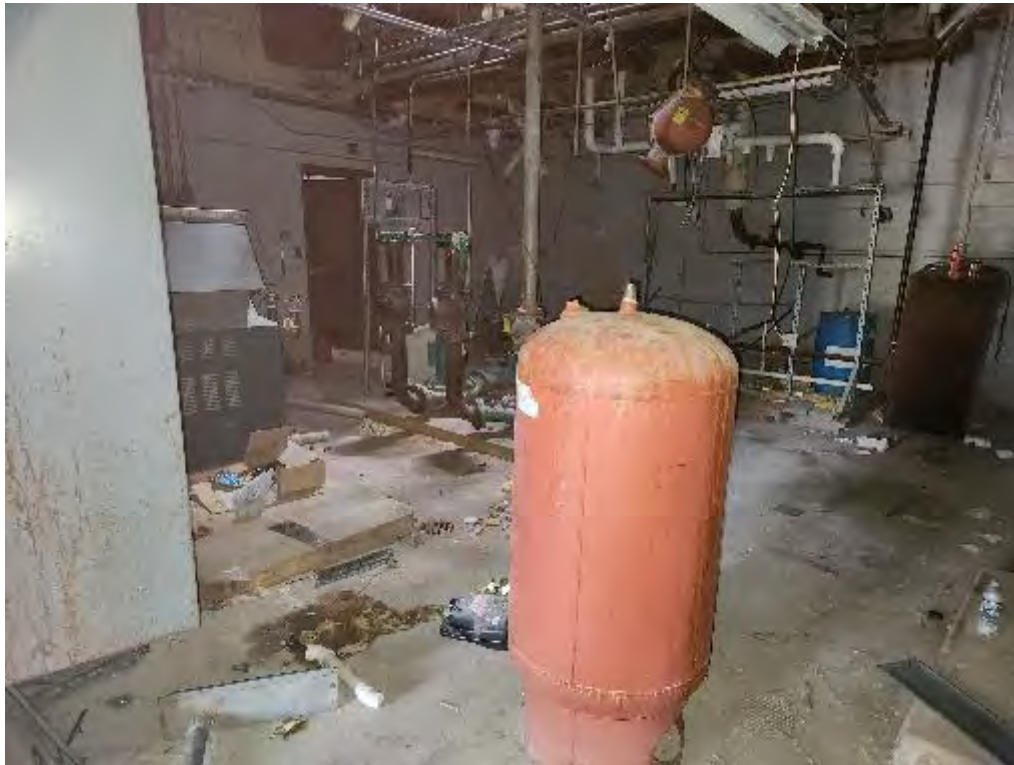
Photograph 17 (Northeast): View of north side of the boiler room in the main Hospital building.
