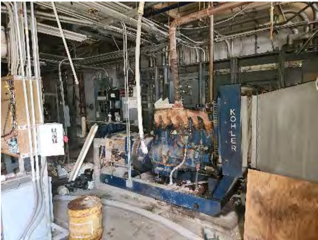
Photograph 16 (NA): View within the boiler room of the main Hospital building.
