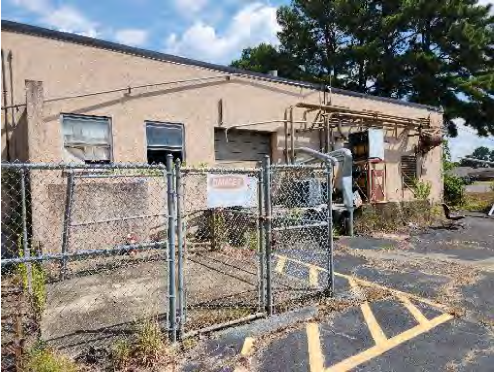
Photograph 15 (Southeast): View of side entrance to the boiler room of the main Hospital building.
