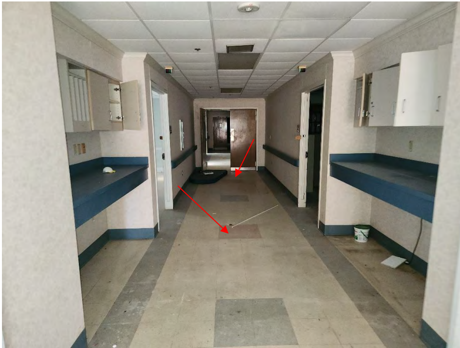
Photo 9: This photograph shows ACM 12- x 12-inch pink with white streaks vinyl floor tile and yellow mastic (HS-VFT09) in the maternity area hallway of the Hospital building (red arrows).
