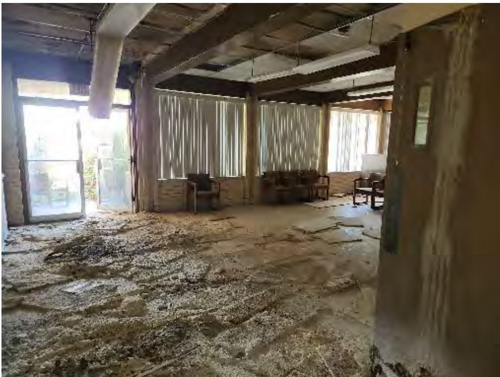
Photograph 18 (Southeast): View of front entryway in the Medical Clinics building. The majority of ceiling tiles had fallen to the floor because of roof leaks.
