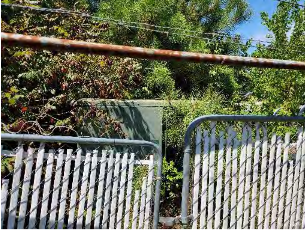
Photograph 37 (West): View of generator within the fenced off area of the Hospital building in the central southwest corner of the subject property.
