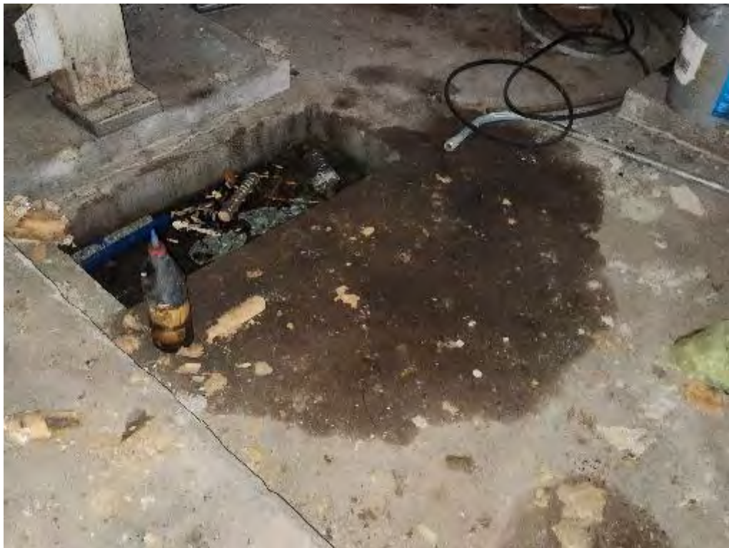
Photograph 22 (NA): View of stained concrete slab next to the air compressor in the boiler room.
