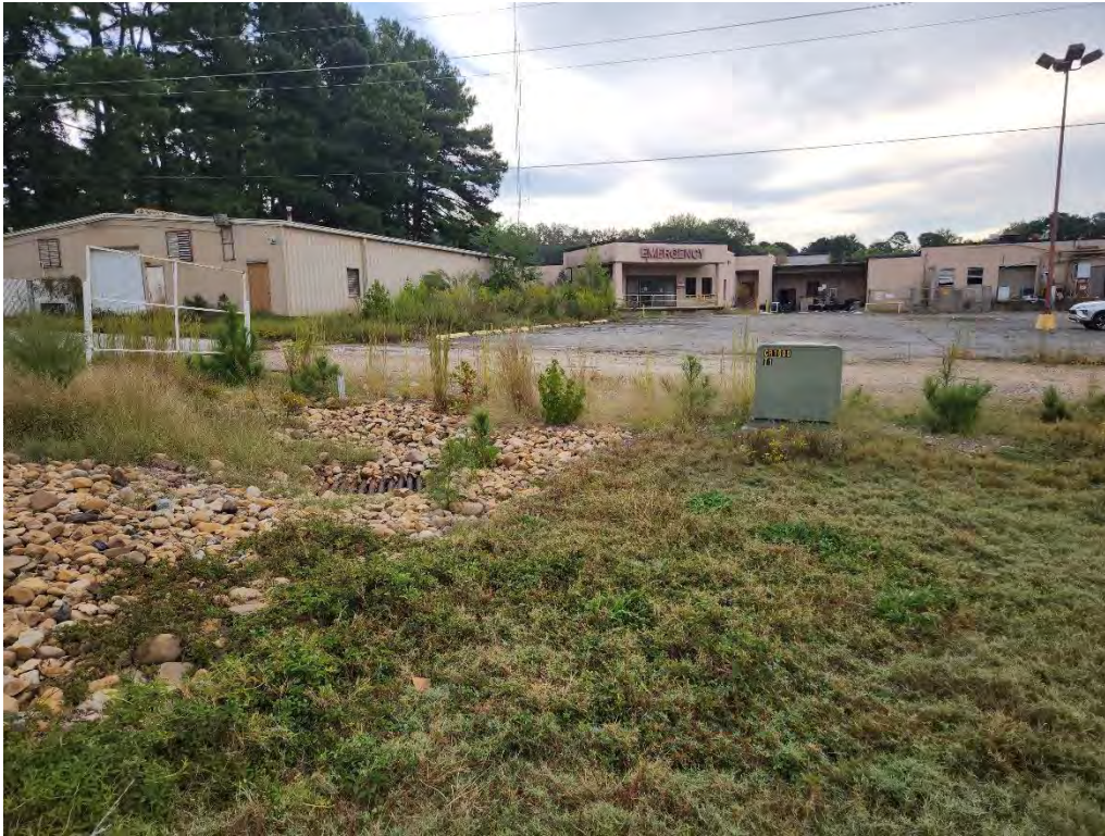
Photograph 33 (East): View of one of the pad-mounted transformers in the northern portion of the subject property.
