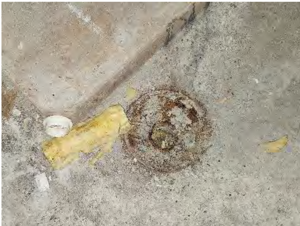
Photograph 26 (NA): View of drains observed throughout the floor of the boiler room in the main Hospital building.
