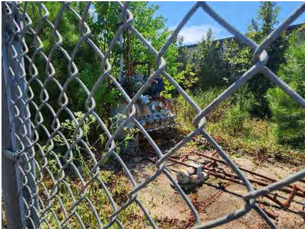
Photograph 36 (Southeast): View of equipment for the generator within the fenced off area of the Hospital building.
