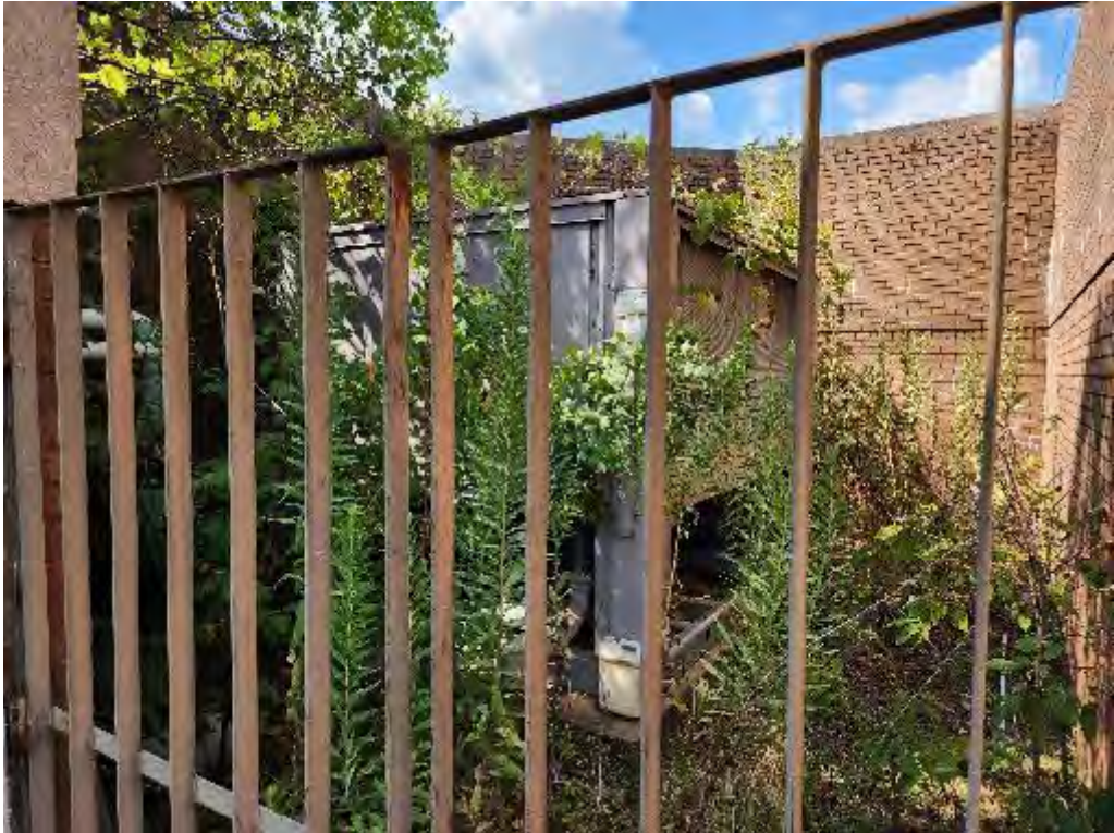
Photograph 33 (West): View of generator on the east side of the Hospital building.
