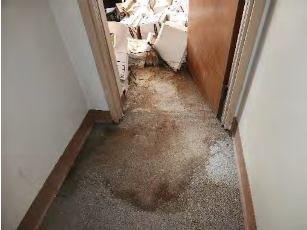
Photograph 11 (Not Applicable [NA]): Overview of water damage leading to the back room.
