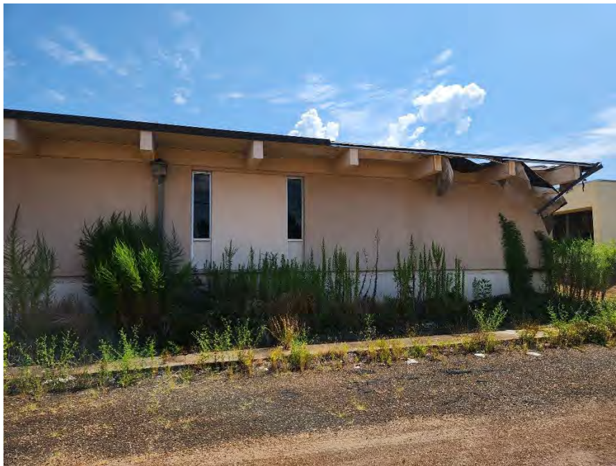
Photo 6: This photograph shows a view of assumed ACM roofing material on the Medical Clinics building.
