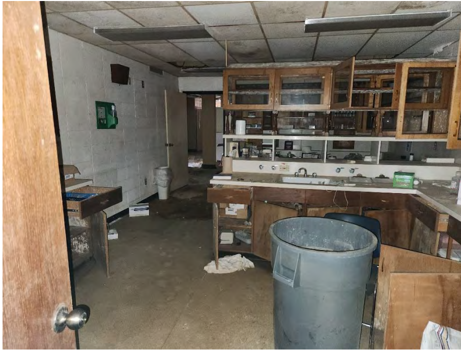
Photo 5: This photograph shows ACM cream sheet vinyl flooring and white mastic (MC-SV02) found in the laboratory room and rooms off the main hallway of the Medical Clinics building.
