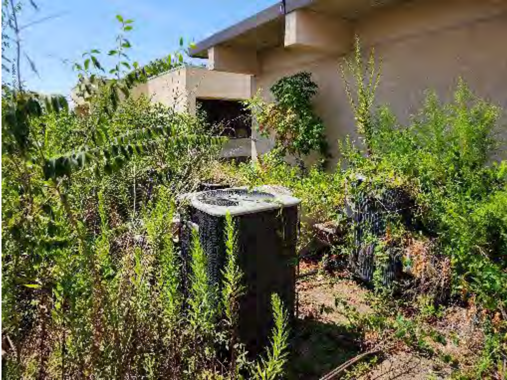
Photograph 25 (Southwest): View of air conditioning units overgrown with vegetation in front of the Medical Clinics building (east side).
