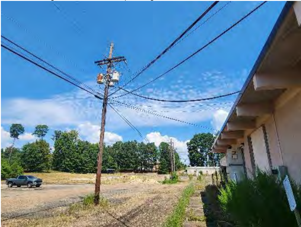
Photograph 14 (North): View of pole-mounted transformer behind the Medical Arts building. North 14 th Street is visible on the left.
