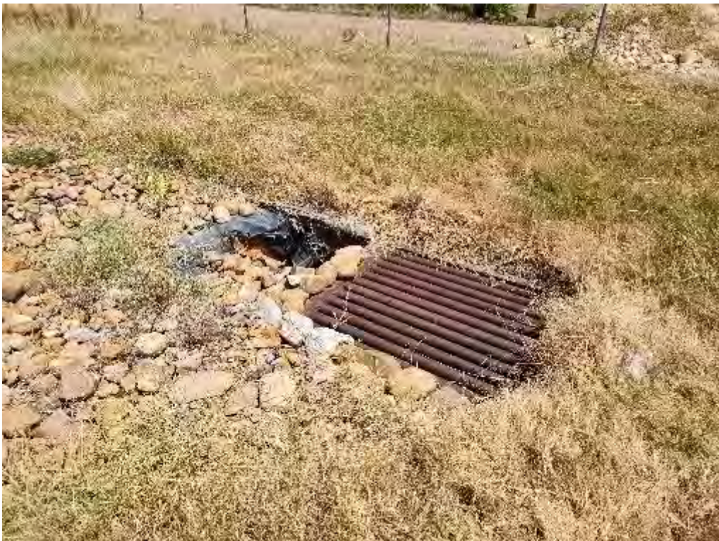
Photograph 32 (Northeast): View of rain runoff drain near the helicopter landing pad.
