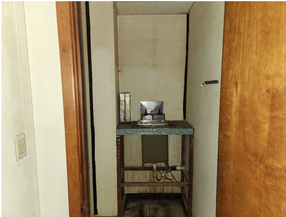
Photograph 41 (North): View of the photo-processing room found in the back of the Medical Arts building, with staining on the floor.
