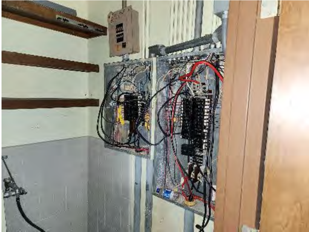
Photograph 13 (NA): View of open electrical paneling seen throughout the main Hospital building.
