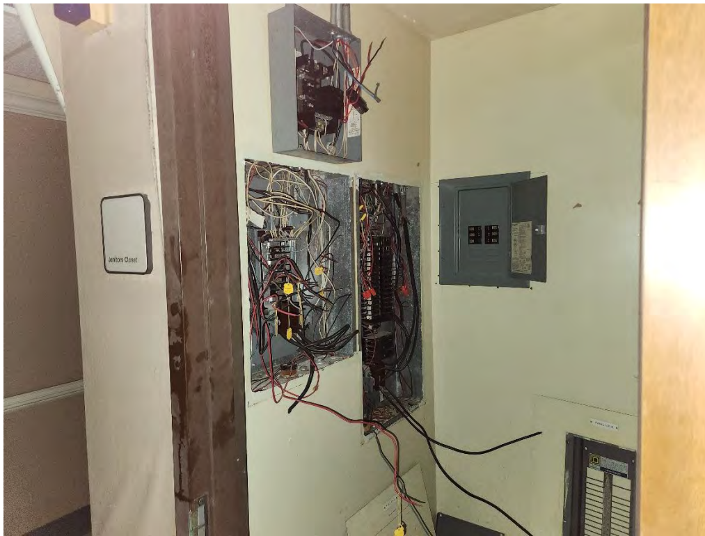
Photograph 9 (NA): View of a broken and stripped breaker box in the Hospital building, typical of the disrepair of most of the breaker boxes observed at the subject property.
