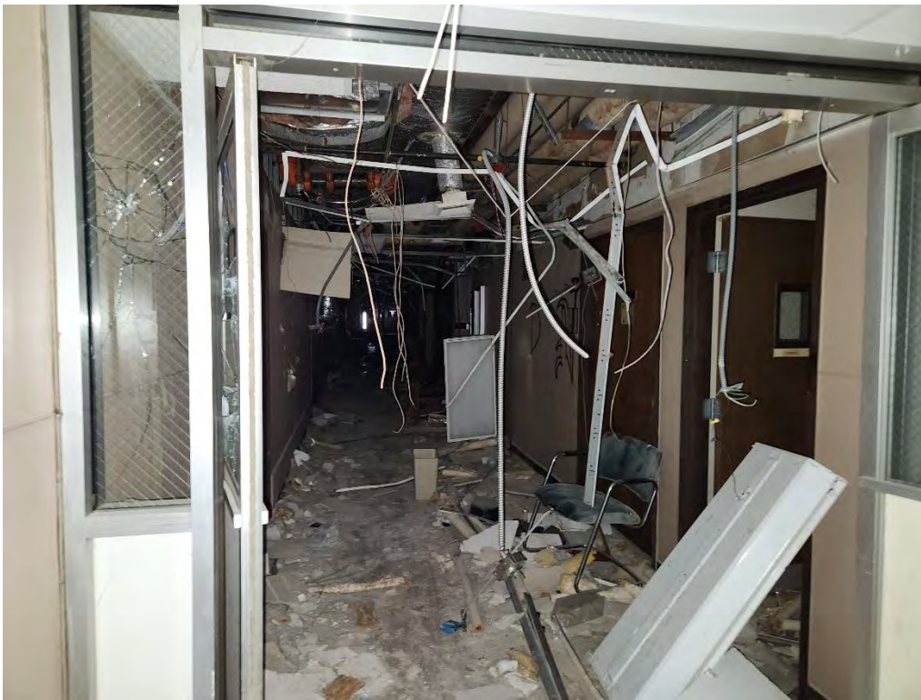
Photograph 5 (West): View of a hallway in the Hospital building, typical of the disrepair observed in most of the hallways in the Hospital building.
