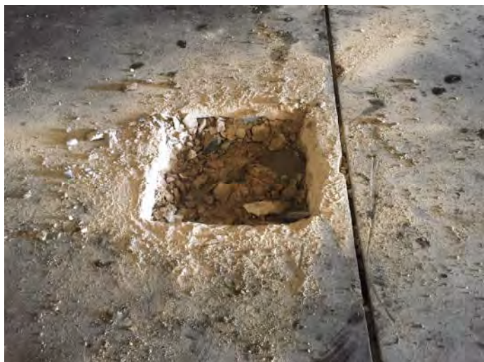
Photo 3. Void space for flush-mount surface completion, MW-2.
