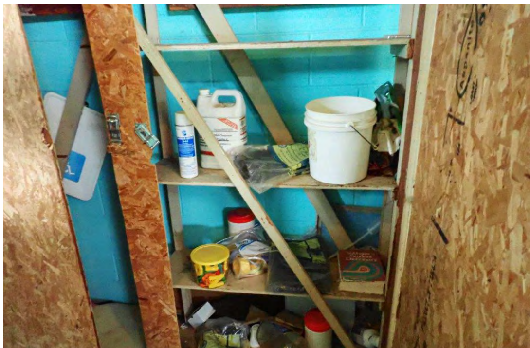
Photograph 22. Classroom building #7380 small containers present in boiler room
