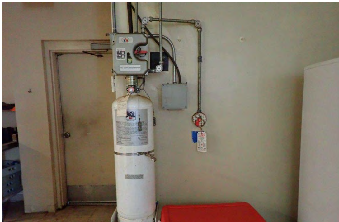
Photograph 30. Cafeteria building #7381 view of kitchen fire suppression system
