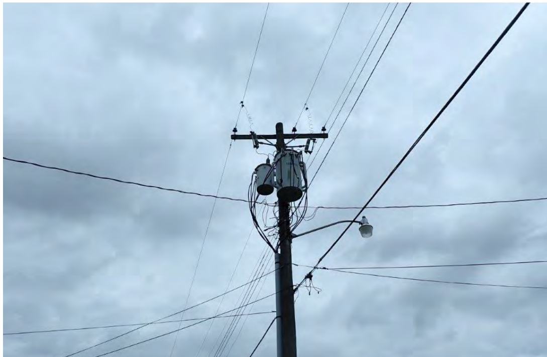
Photograph 9. Pole mounted transformer located adjacent to Subject Property
