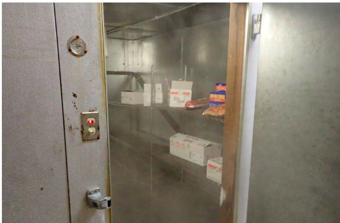
Photograph 28. Cafeteria building #7381 view of walk-in freezer
