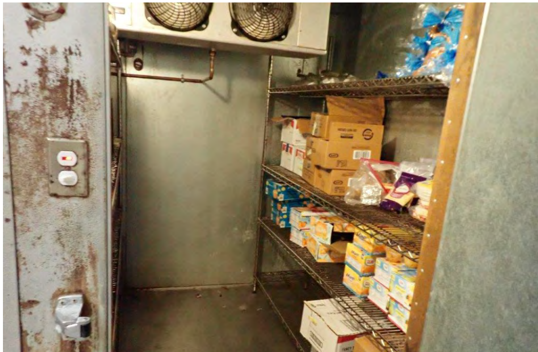
Photograph 29. Cafeteria building #7381 view of walk-in cooler
