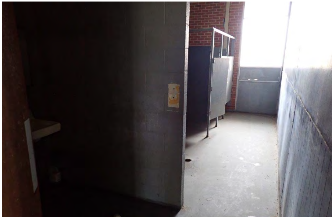
Photograph 19. Classroom building #7380 view of boys bathroom
