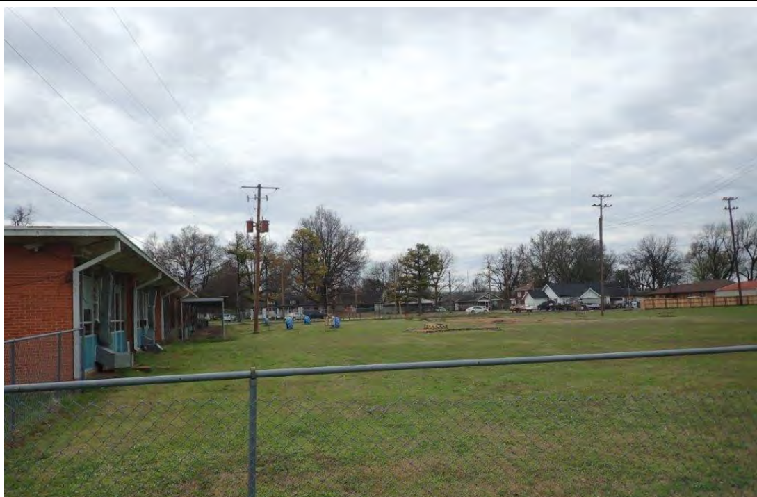
Photograph 10. Pole mounted transformer adjacent to classroom building #7380
