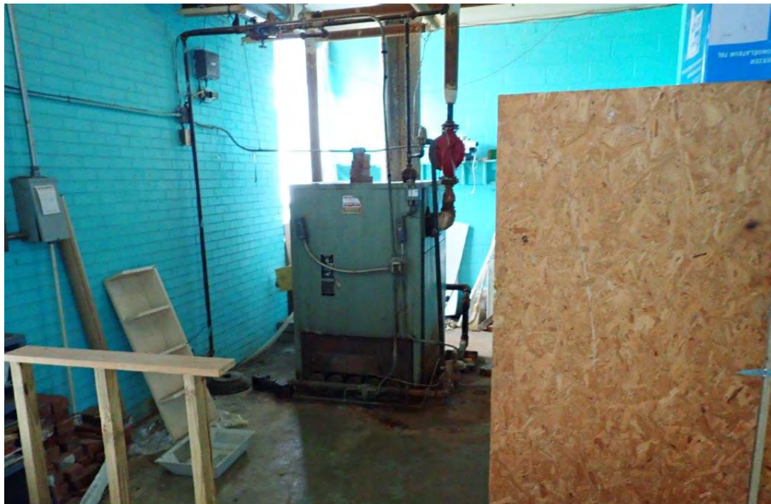
Photograph 21. Classroom building #7380 view of boiler room
